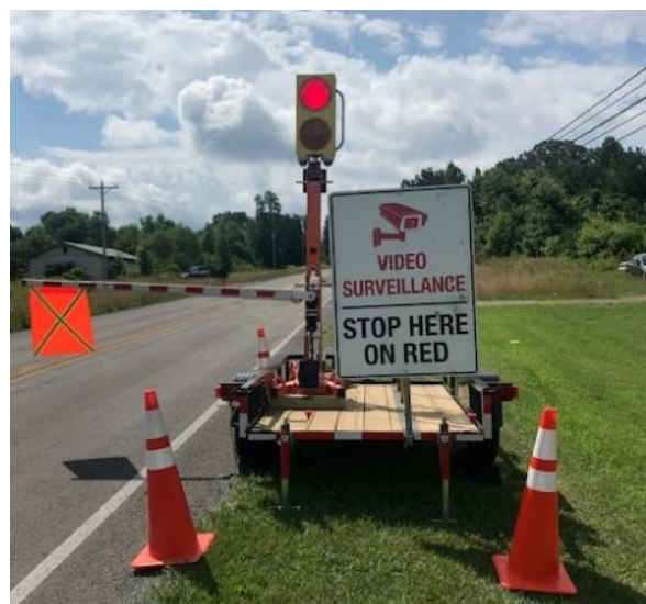
Figure 12. AFAD with Video Monitoring in Alabama
