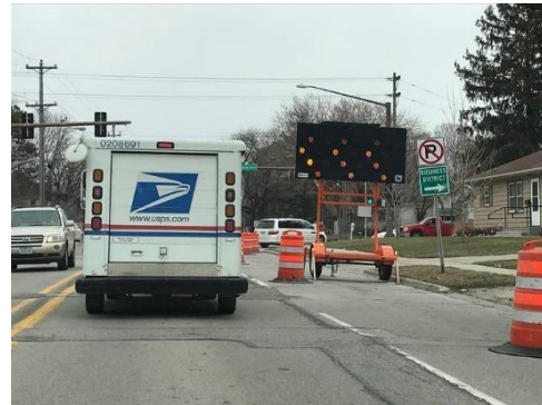
Figure 7. Arrow Board Field Location Example
