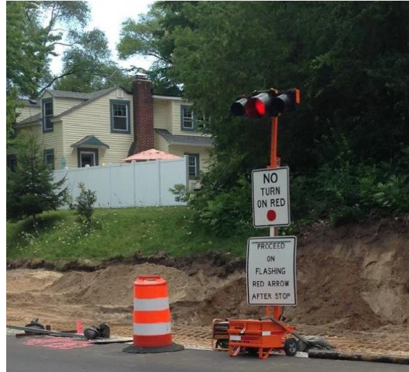
Figure 10. DAD Installed on M-44 in Michigan
