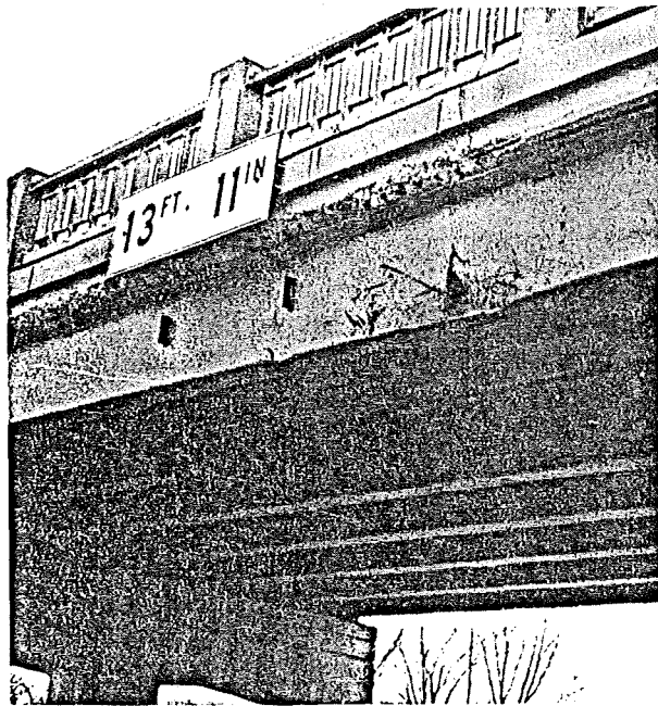
Figure 1a. East fascia of damaged span showing impact point of the fork-lift.
