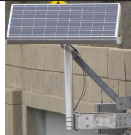
Communication Base Station
