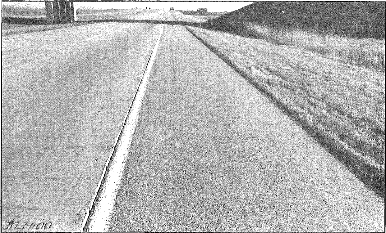
Figure 4. Showing the typical condition of the experimental bituminous shoulders in the fall of 1984 (project 1).
