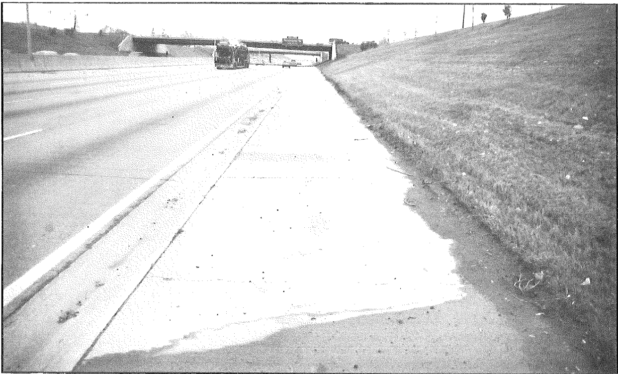
Figure 7. Showing the typical condition of the experimental concrete shoulders in the fall of 1984 (project 20).
