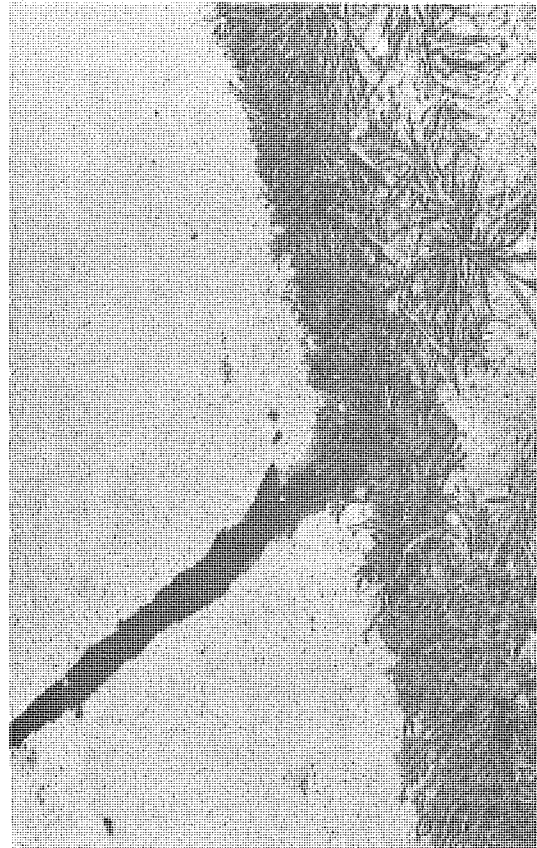
Figure 4. Three-year-old base plate; Project 39-40, C4; constr. 1953.
