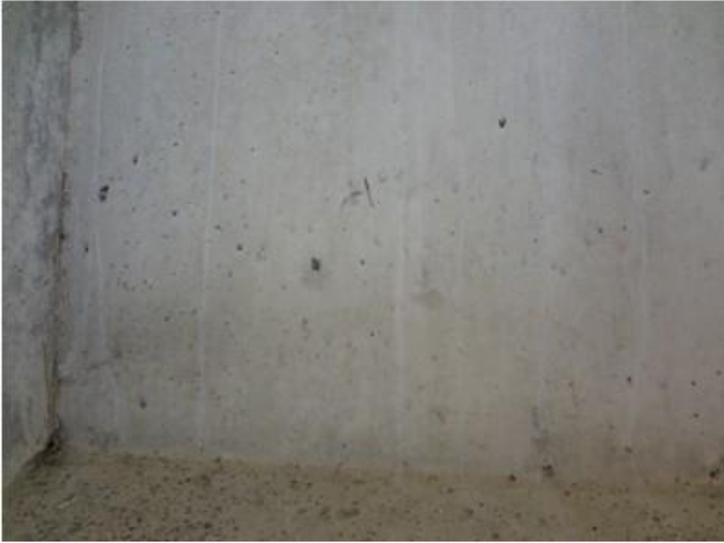
Figure A42. Cracks on exterior girder on east side, west face, north abutment (#1829).
