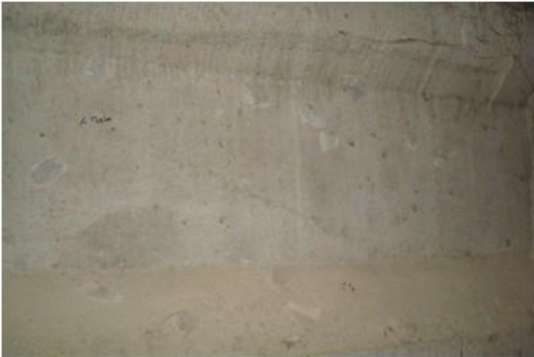
Figure A74. Cracks on Girder 5 th from west side, west face, south abutment (#12693).
