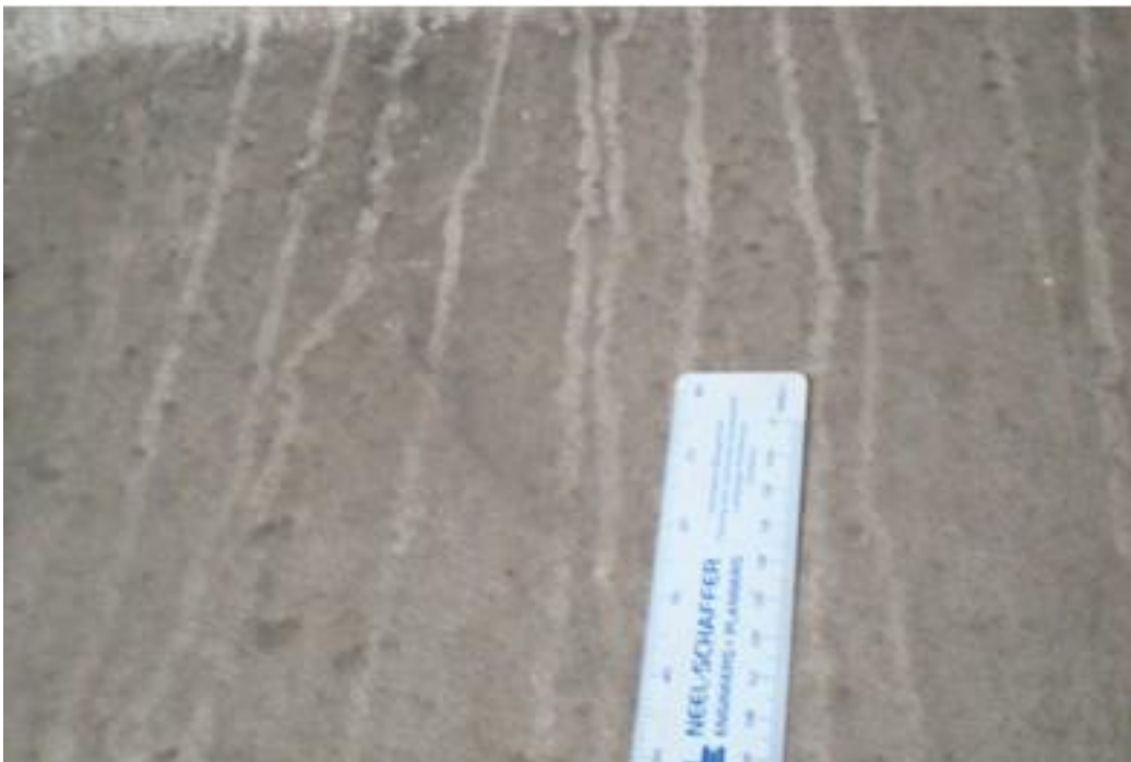
Figure A10. Cracks on south span girder, north end, 5 th beam from east side, east face (#7933).
