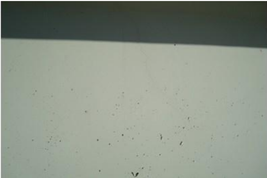
Figure A47. Cracks on exterior girder, west side, west face, south abutment (#1829).
