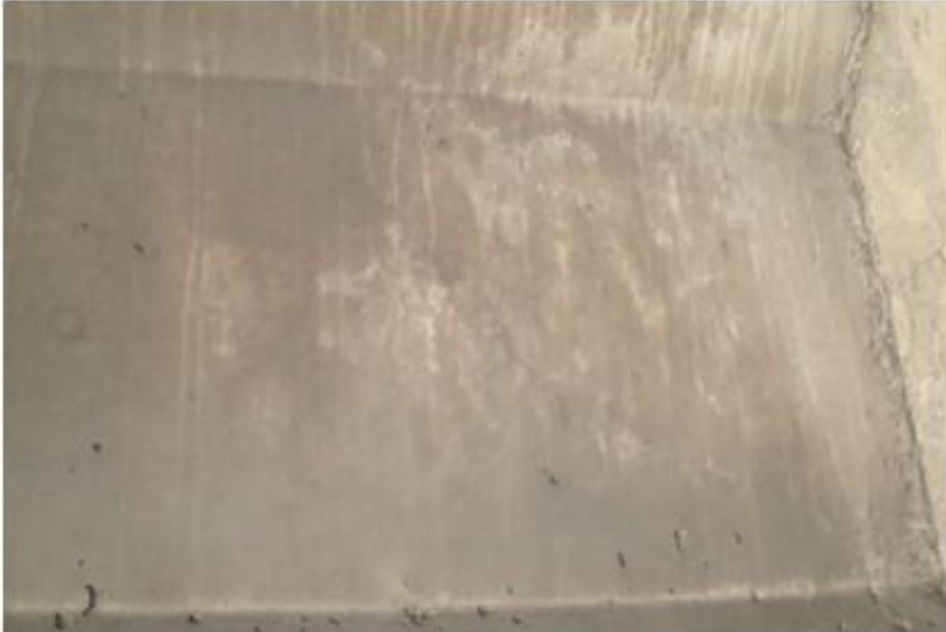
Figure A28. Cracks on south span girder, 6 th beam from west side, west face, south abutment (#7933).
