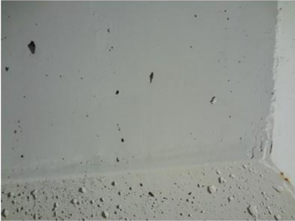
Figure A40. Cracks on exterior girder on east side, east face, north abutment (#1829).
