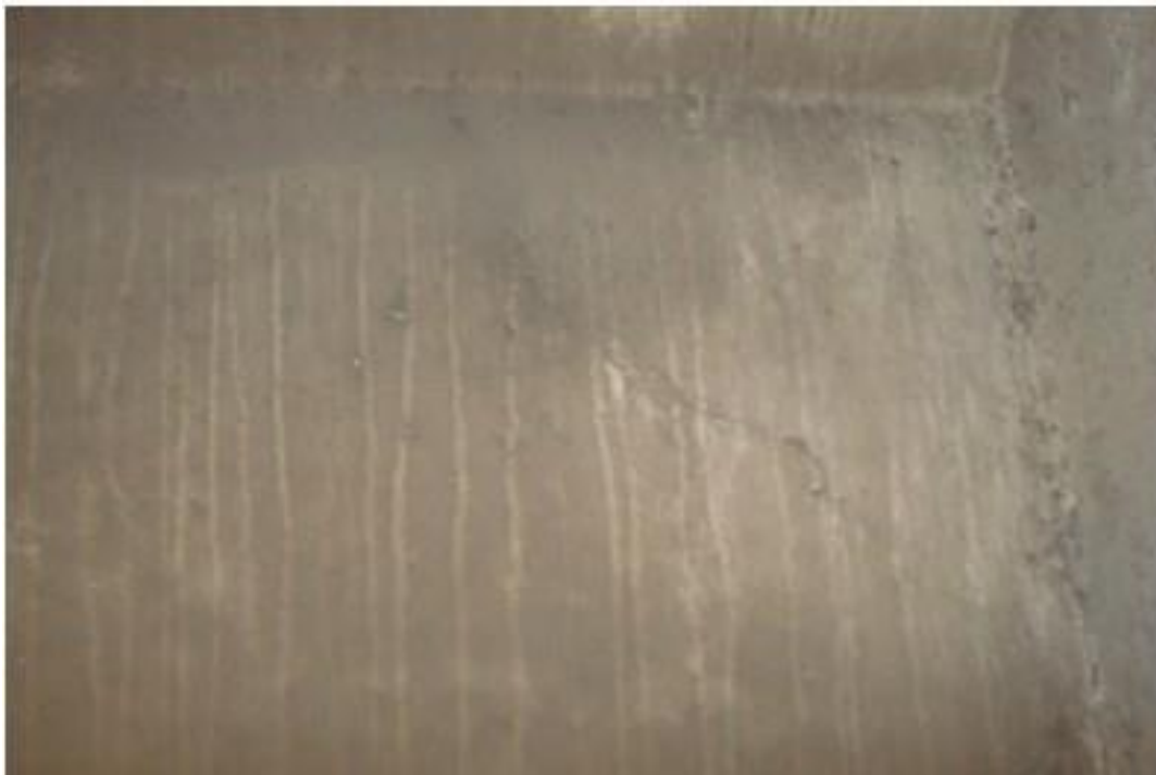
Figure A32. Cracks on south span girder, 4 th beam from east side, west face, south abutment (#7933).
