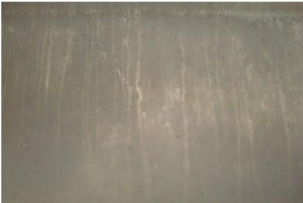
Figure A34. Cracks on south span girder, 3 rd from east side, west face, south abutment (#7933).
