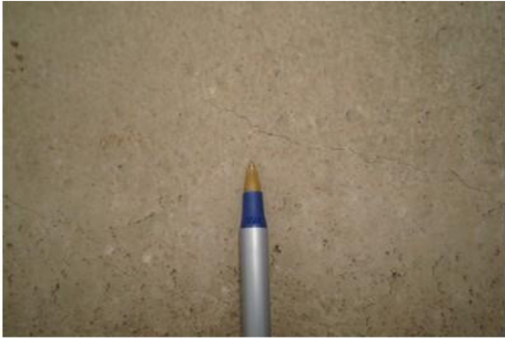
Figure A71. Cracks on exterior girder, west side, west face, south abutment (#9728).
