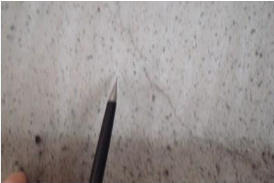
Figure A3. Cracks, exterior girder of north span, south end, east side, interior face (#7933).
