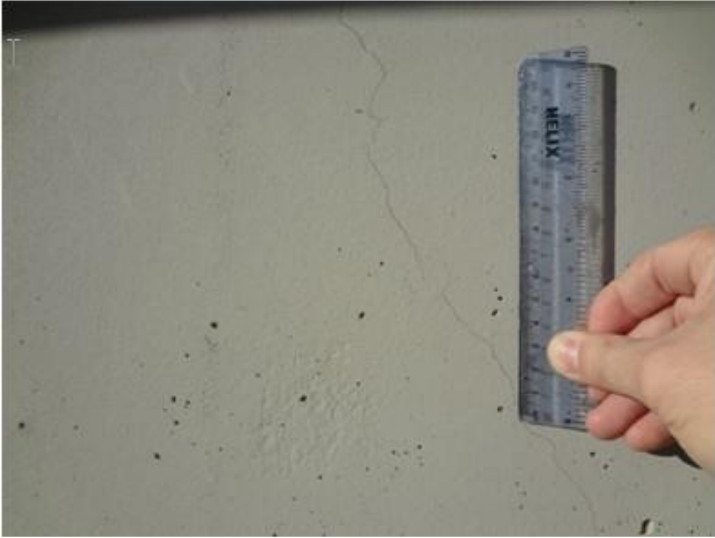
Figure A51. Cracks on east-most exterior girder, east face, north abutment (#1830).
