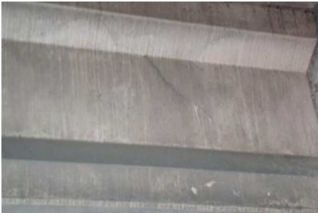
Figure A13. Cracks on south span girder, north end, 4 th beam from east side, east face (#7933).
