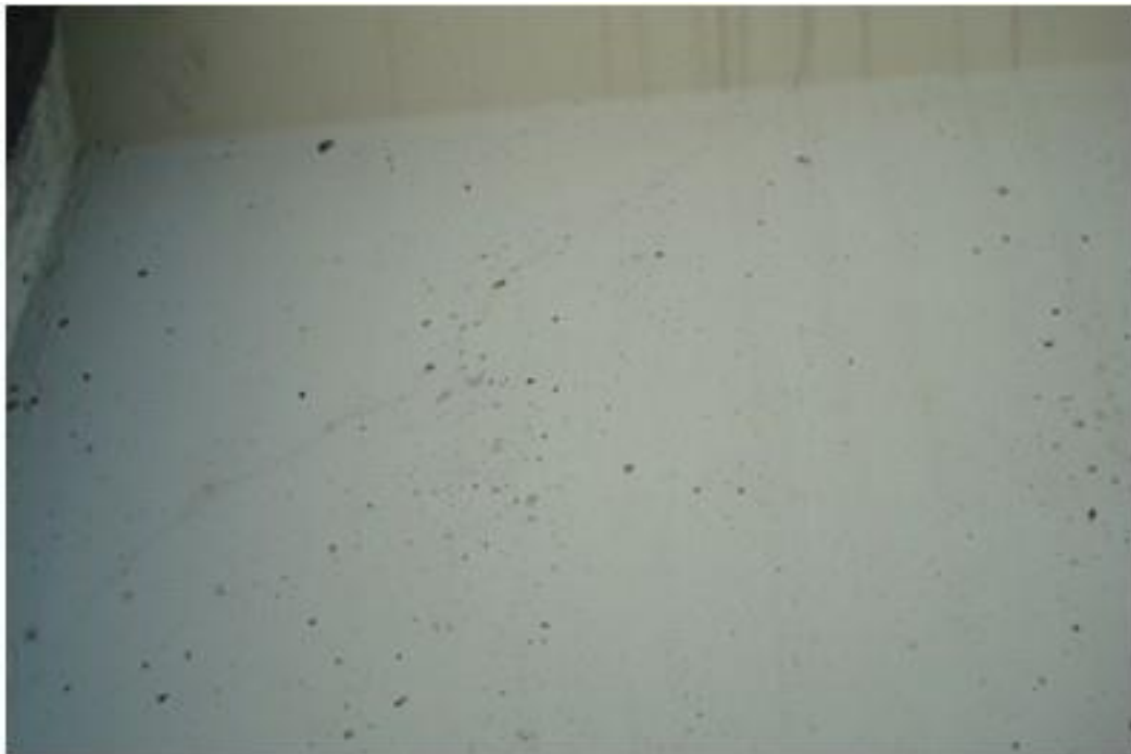
Figure A24. Cracks on north span, exterior girder on west side, west face, north abutment (#7933).
