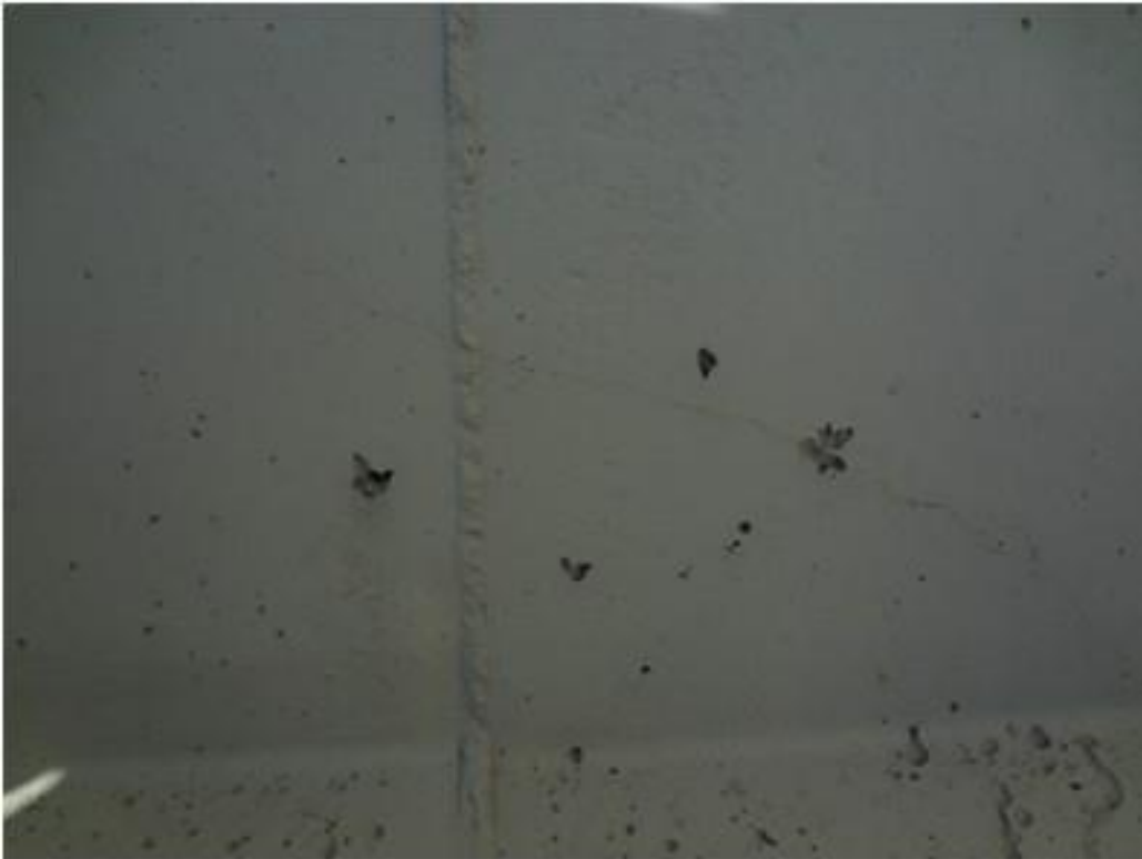
Figure A53. Cracks on girder 4 th from east side, east face, north abutment (#1830).
