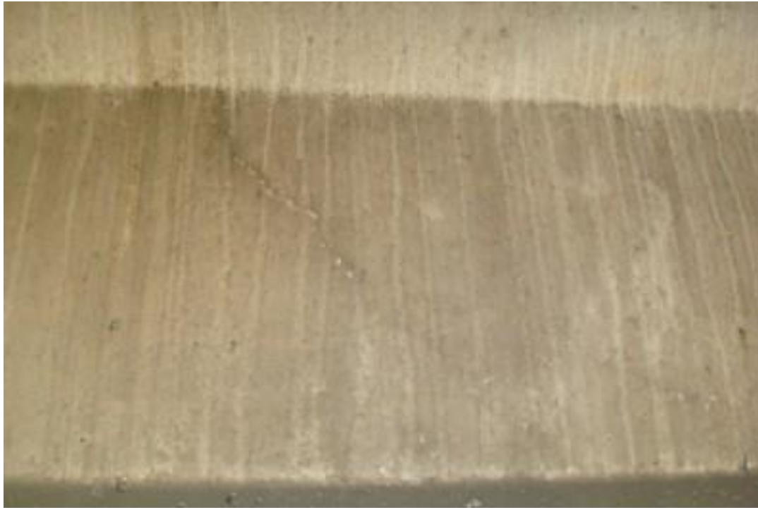
Figure A8. Cracks on south span girder, north end, 6 th beam from east side, east face (#7933).
