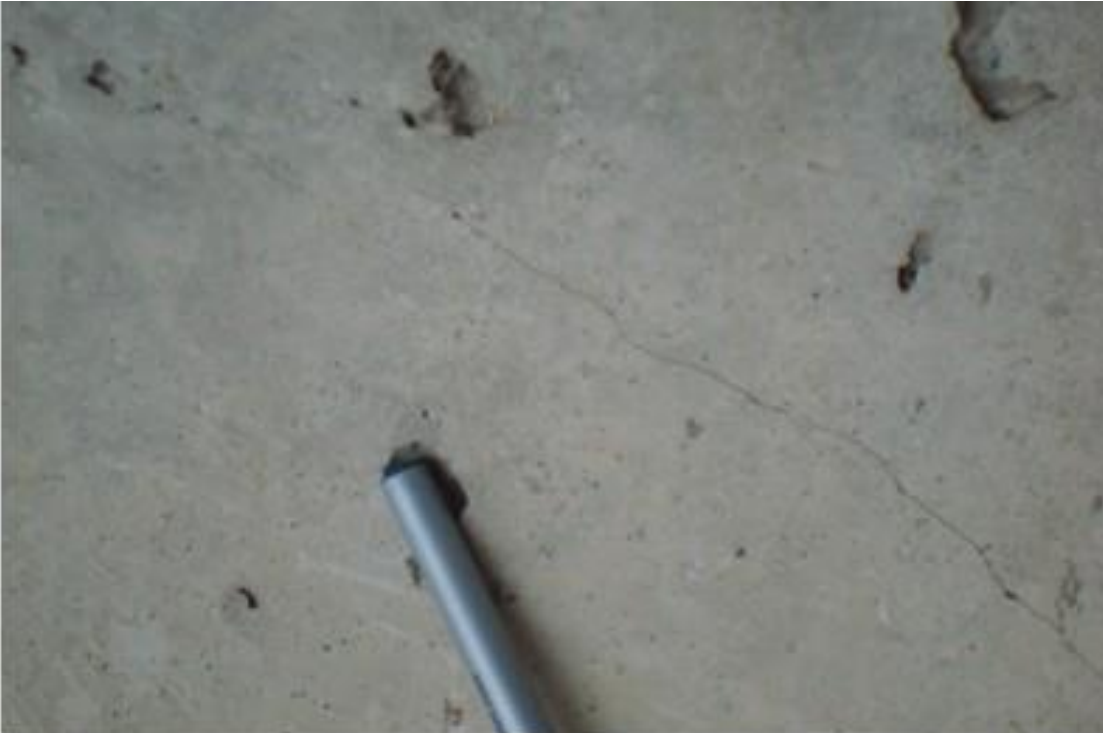
Figure A67. Cracks on exterior girder, east side, east face, north abutment (#9728).
