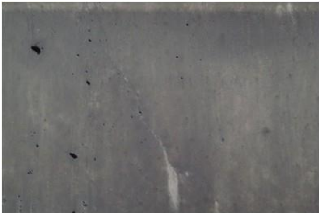
Figure A22. Cracks on north span girder, 2 nd beam from east side, east face, north abutment (#7933).
