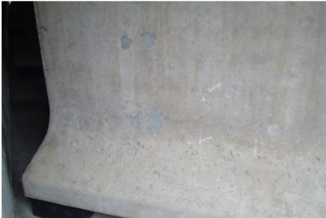
Figure A65. Cracks on exterior girder, west side, west face, north abutment (#9728).
