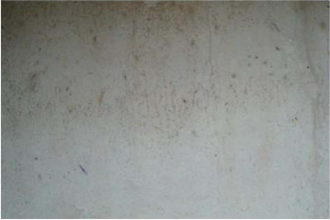
Figure A69. Cracks on exterior girder, east side, east face, south abutment (#9728).
