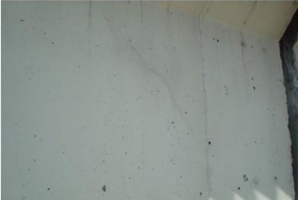
Figure A18. Cracks on south span girder, exterior beam, west side, exterior face (#7933).
