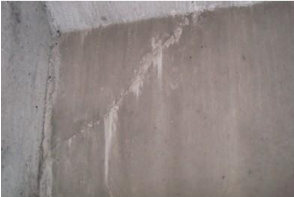
Figure A20. Cracks on north span girder, exterior beam, east face, north abutment (#7933).
