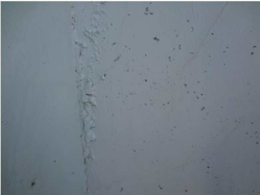
Figure A59. Cracks on exterior girder on west side, west face, north abutment (#1830).
