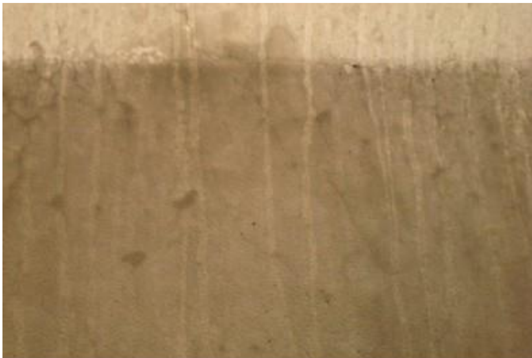
Figure A15. Cracks on south span girder, north end, 2 nd beam from east side, east face (#7933).
