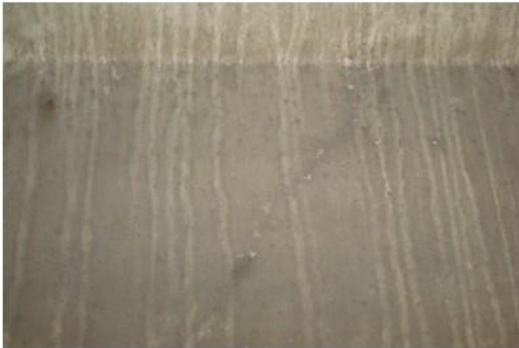
Figure A7. Cracks on south span girder, north end, 6 th beam from east side, west face (#7933).
