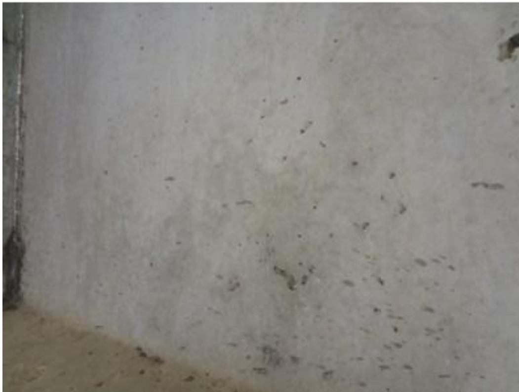
Figure A55. Cracks on girder 3 rd from east side, west face, north abutment (#1830).
