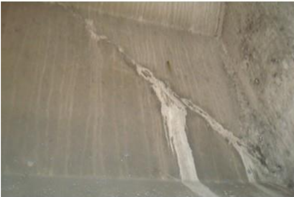
Figure A26. Cracks on south span girder, 3 rd beam from west side, west face, south abutment (#7933).
