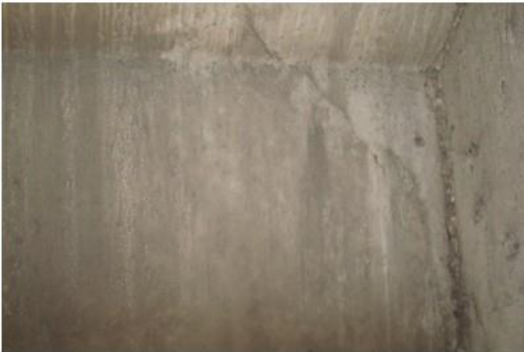
Figure A37. Cracks on south span, exterior girder, east side, interior face, south abutment (#7933).
