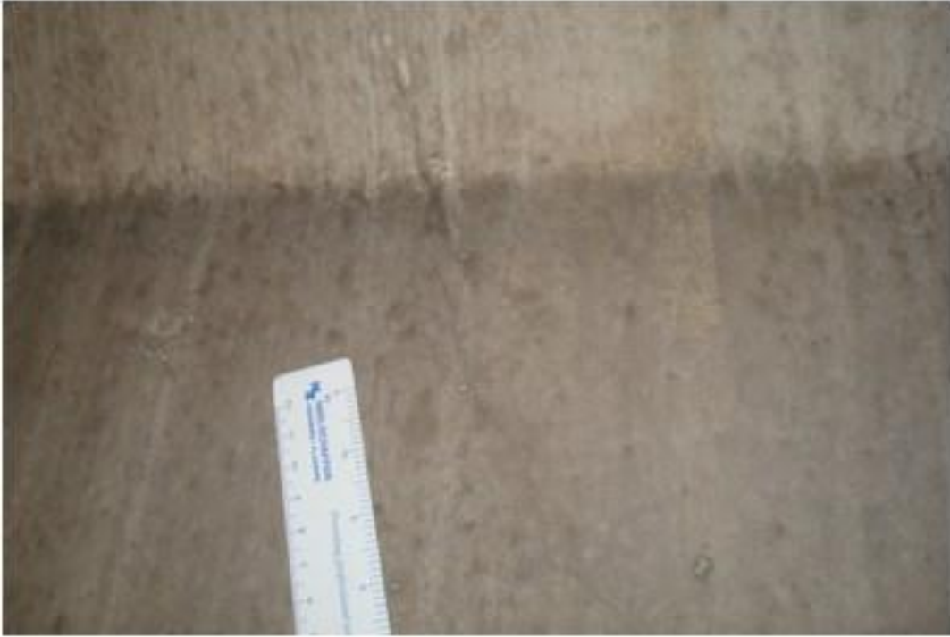
Figure A5. Cracks, girder at south span, north end, 4 th beam from west side, west face (#7933).
