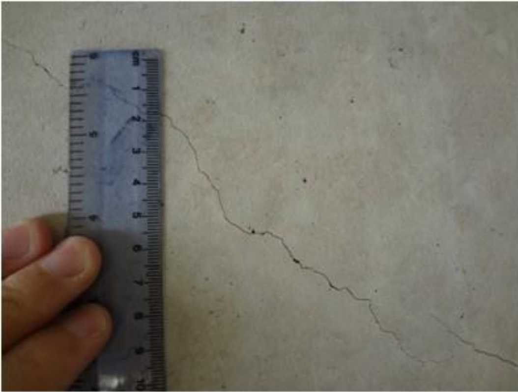
Figure A57. Cracks on girder 2 nd from west side, east face, north abutment (#1830).
