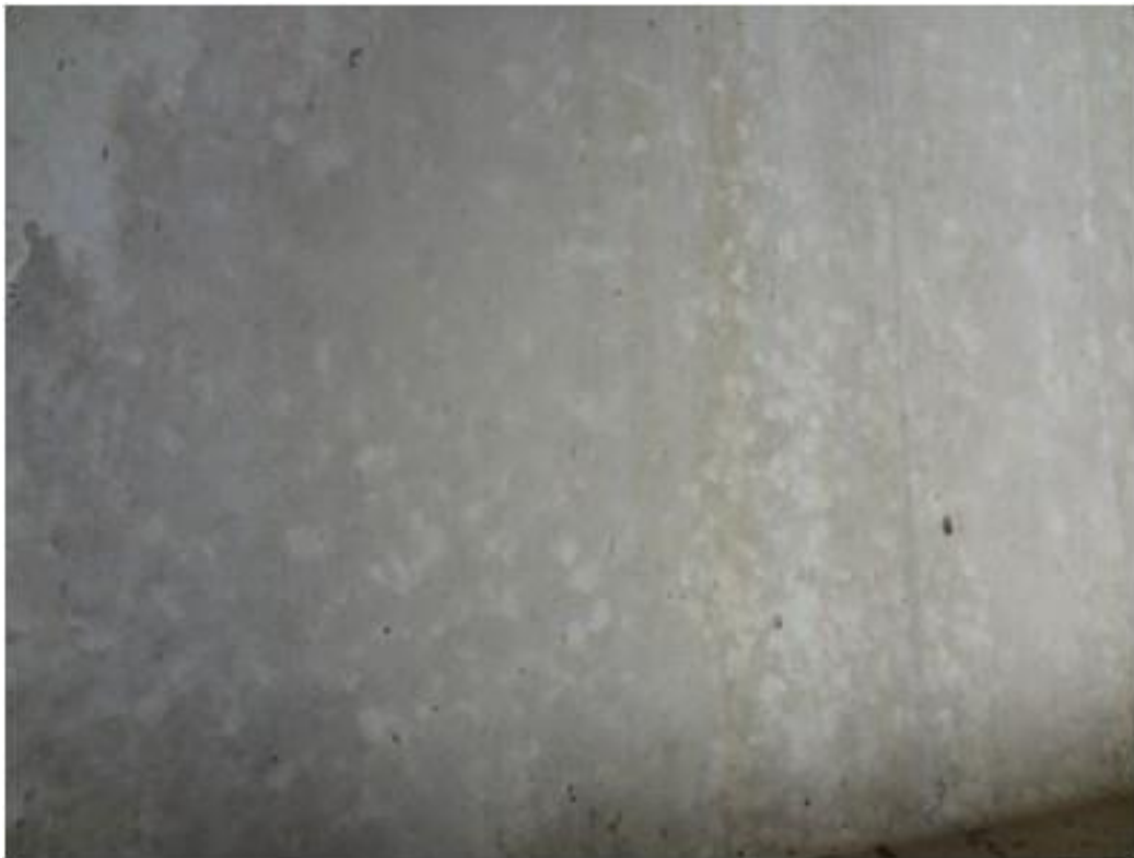
Figure A44. Cracks on girder 2 nd from east side, east face, north abutment (#1829).
