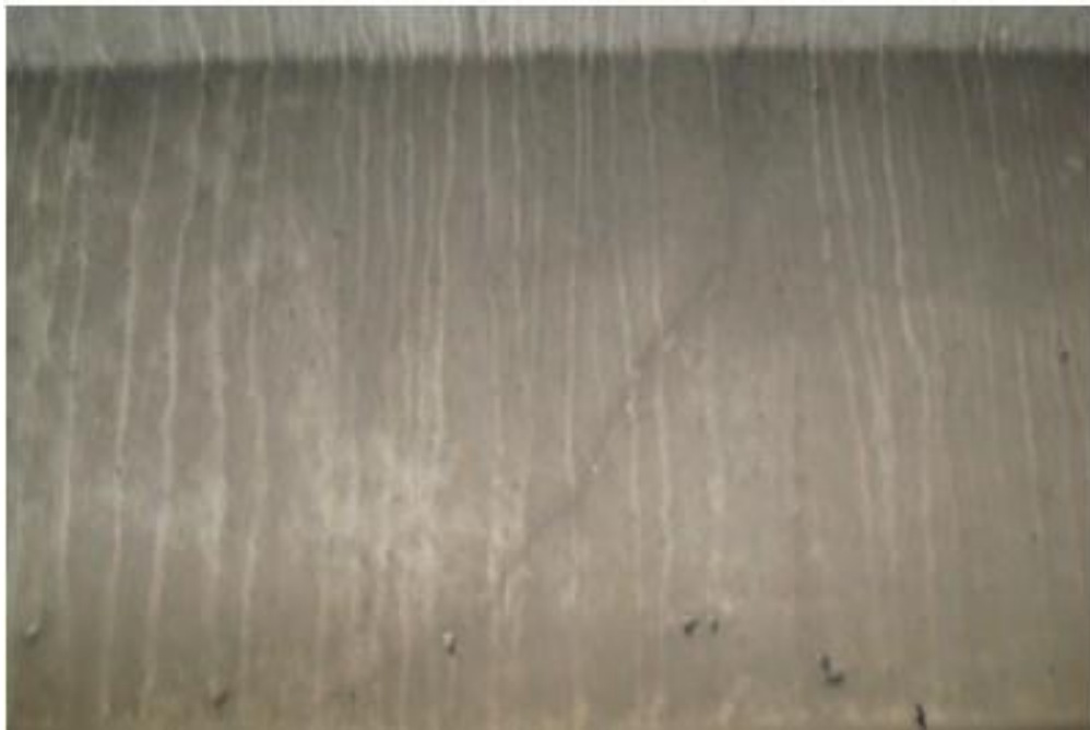
Figure A30. Cracks on south span girder, 7 th beam from west side, east face, south abutment (#7933).
