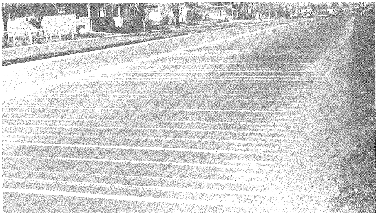
Figure 3. Poor durability of Detroit stripes after six months of exposure (below). Stripes were deposited in duplicate--beaded and unbeaded.
