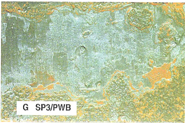
Figure 15 - Painting system applied over mill scale, power tool cleaned by power wire brush.
