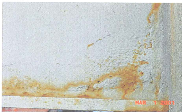
Figure 14 - Corrosion on the east fascia beam at the abutment of span 1 after 40 months
