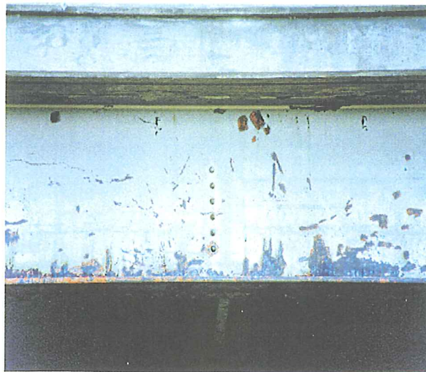
Figure 11 - Cedar St fascia after power tool cleaning
