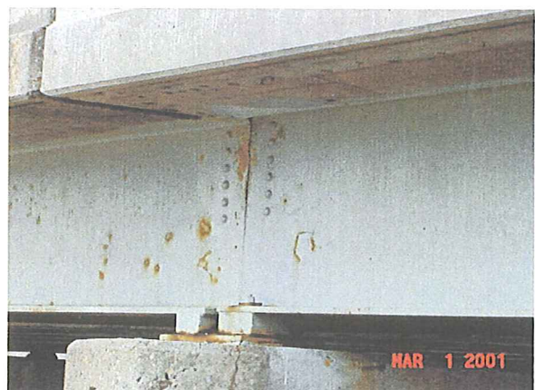
Figure 8 - West fascia over pier 1 after 4 1/2 years
