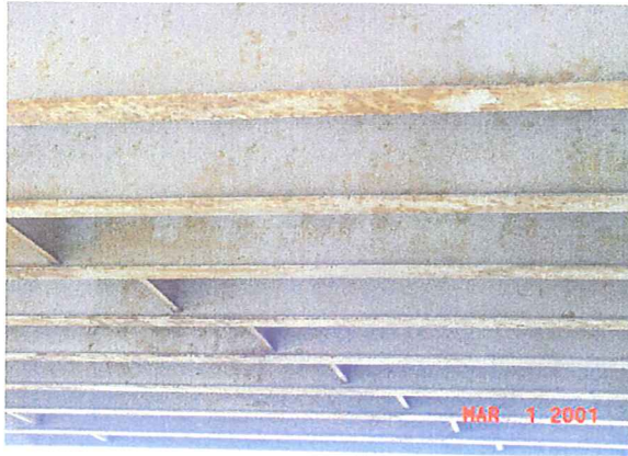
Figure 9 - Over WB traffic lanes after 4 1/2 years
