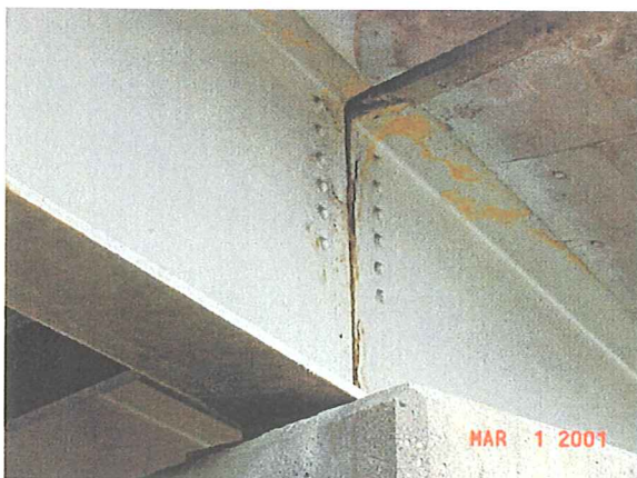
Figure 7 - East Fascia over pier 1 after 4 1/2 years
