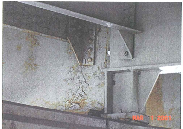
Figure 6 - Beam G @ Pier 1 after 4 1/2 years
