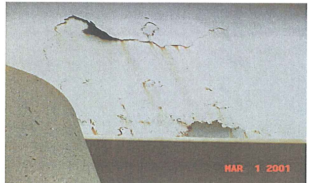
Figure 4- after 5 years (Close up of lifting coating)
