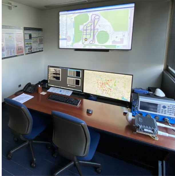
Figure 5: Mcity Traffic Management Center, which is also linked to the City of Ann Arbor traffic control network at 70+ signalized intersections and specialized roadside installations – overlaid on the lower right-hand display.
