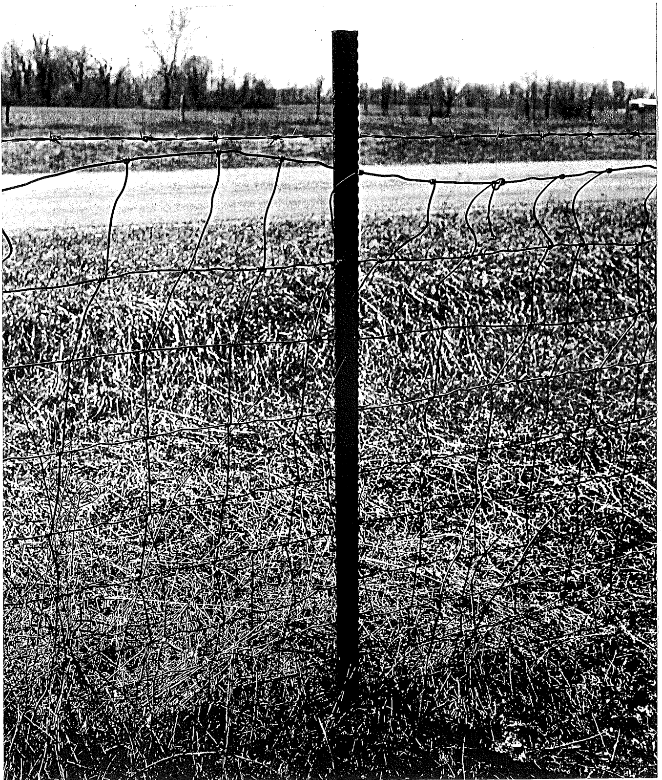
Close-up of post shown in preceding photograph shows that the tie clips are missing.
