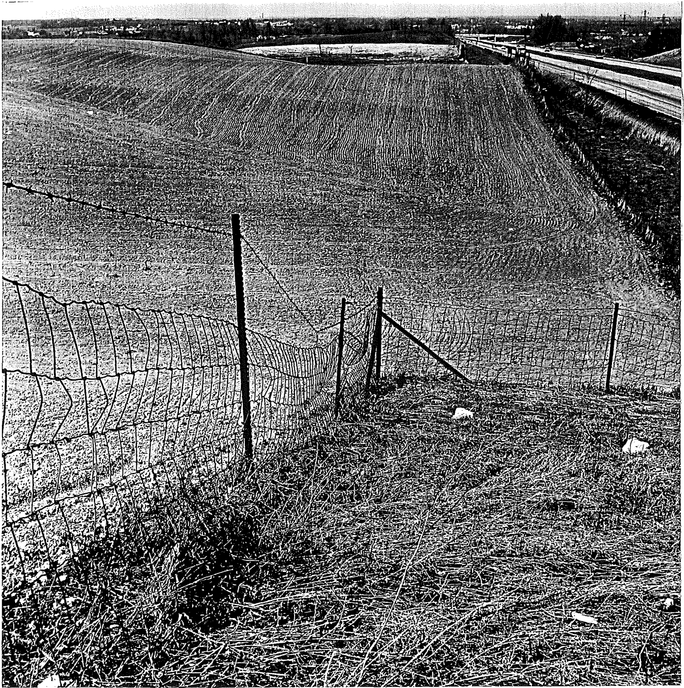
Sagging of fence wire of right-of-way fence on west side of US 131 about 10 miles north of Wayland. Note wire attached to barbed wire holding fence wire up, also type of bulging suggestive of collision with farm machinery.
