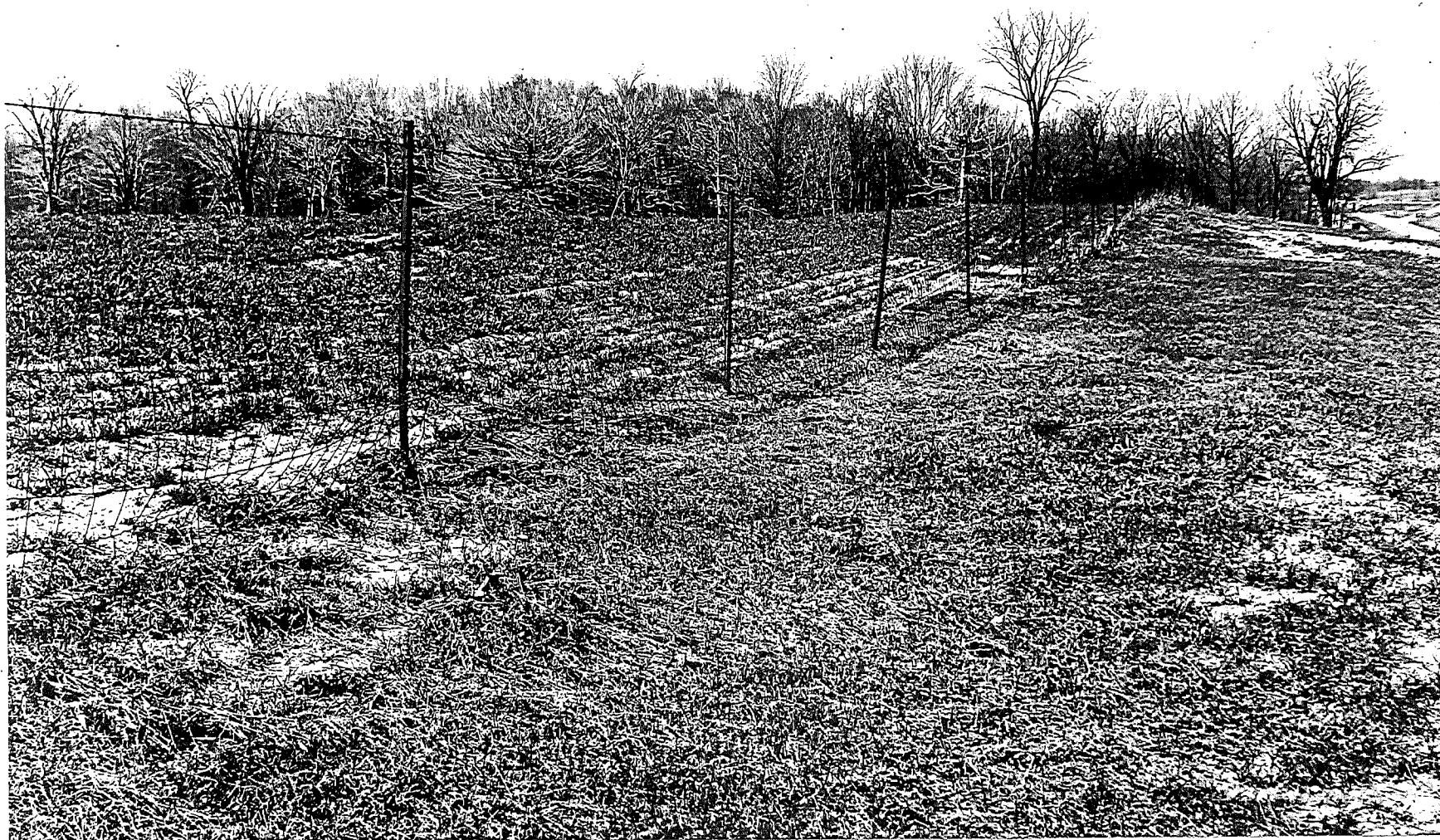
Severe sagging of fence wire involving 8 posts of right-of-way fence on west side of US 131 about 5 miles north of Wayland. Although this damage could have resulted from impact with farm machinery, the gradual contour of the bulges plus the ground slope suggest that movement of heavy snow masses may have been responsible.
