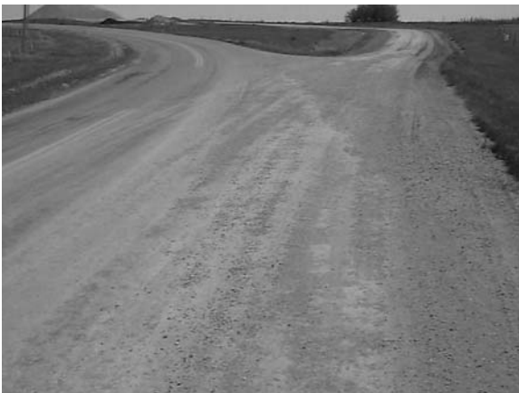
EXHIBIT V-17 Roadway Debris on Curve
