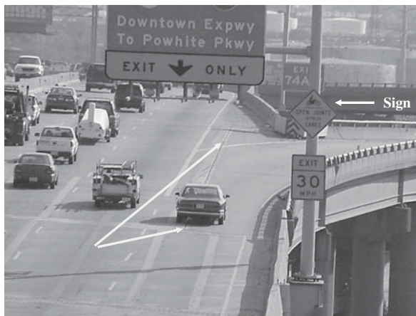
EXHIBIT V-23 Irregular Roadway Surface and Advance Warning Sign
