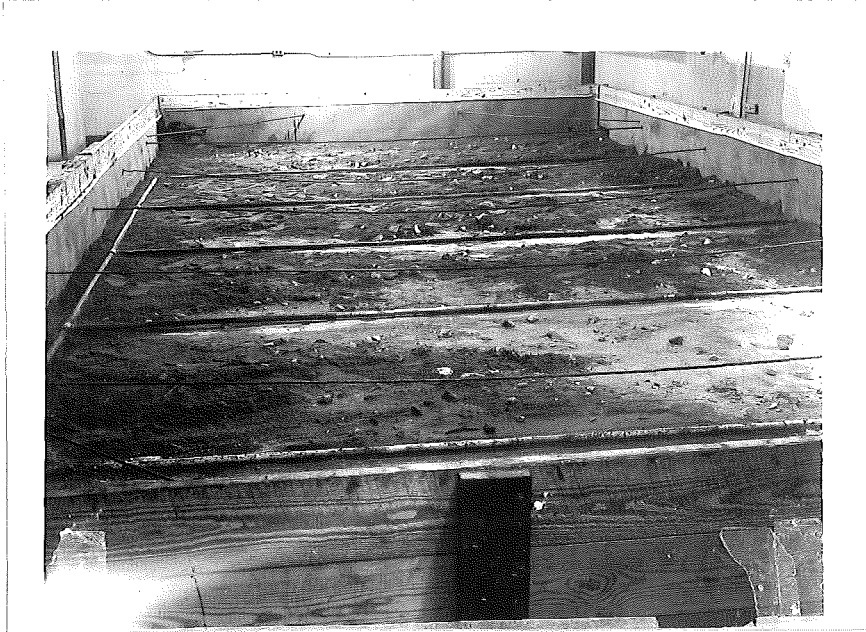
Figure 1. Form for subgrade showing tie rods, waterproofing and moisture control pipe layout.
