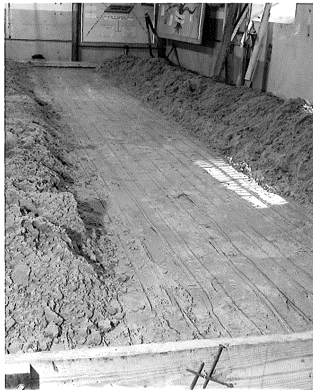
Figure 2. Wire heating grid placed in subgrade to control temperature differential in slab.
