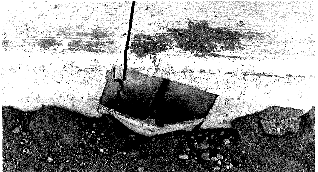
Figure 9. When non-metallic end plates fail to adhere to the slab edge, foreign material freely infiltrates into the joint crack.
