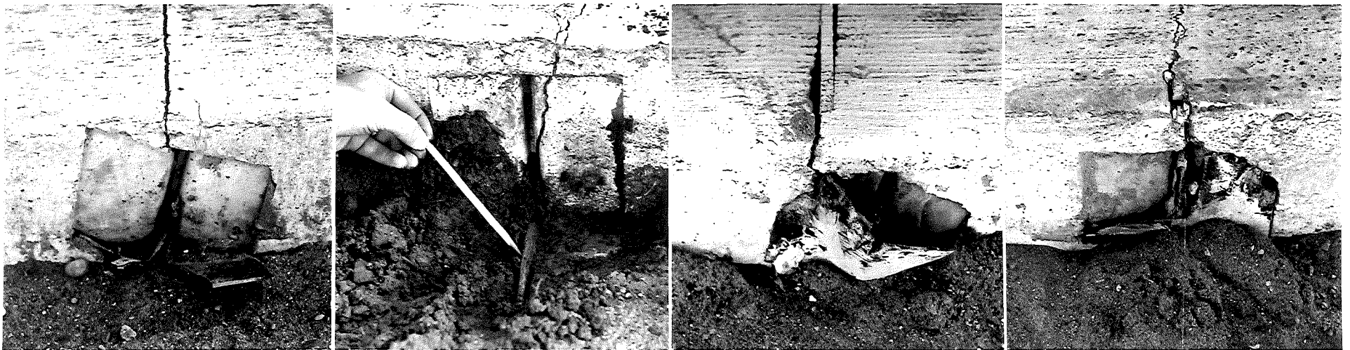
Figure 8. End plates are often torn or otherwise damaged, either during construction or subsequent grading operations.
