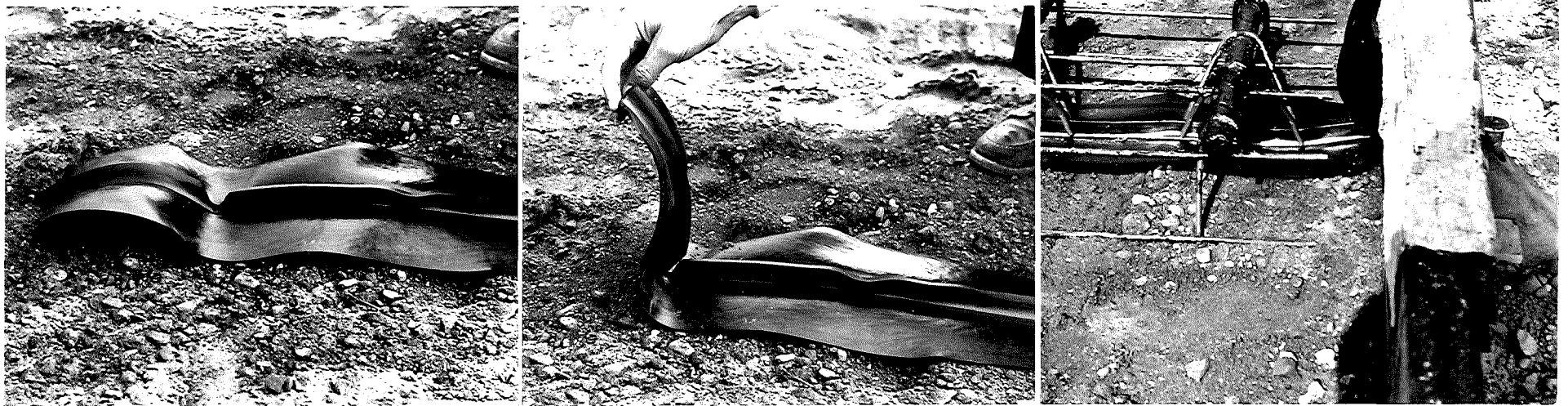
Figure 2. A typical wrinkled base plate, immediately before installation (left). The same plate is shown at center with the end plate turned up, and at right after installation as concrete is being poured.
