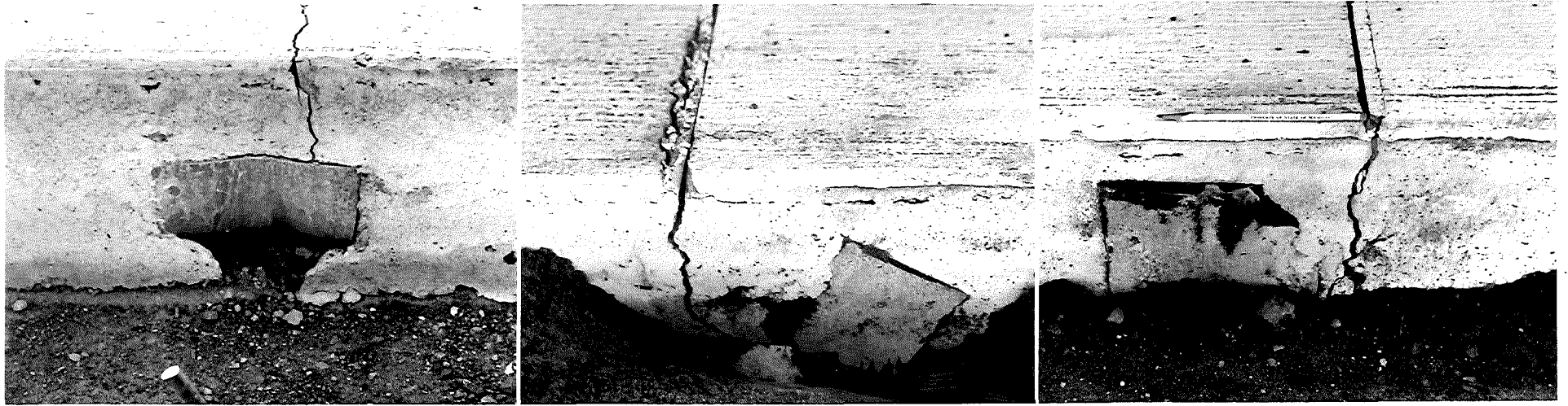
Figure 7. The three most common types of incorrect placement for non-metallic base plates are formation of a curve rather than a right angle at the pavement edge (left); tilting of the plate during pouring operations (center); and misalignment of the top surface joint groove (right).
