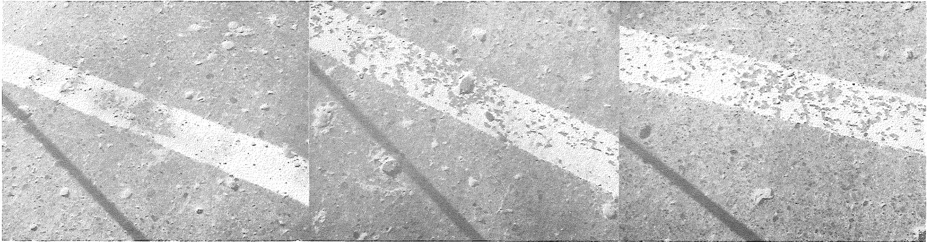
▲ STRIPE 25, NORTH WHEEL TRACK . NORTH LANE, 50% REMAINING. PAINT B
