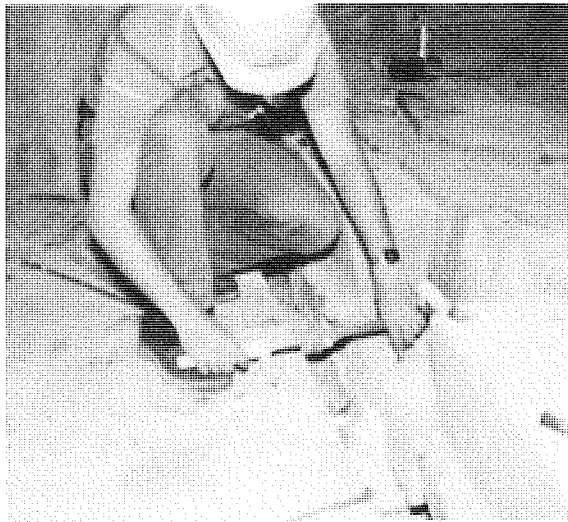
Figure B-18. Measuring opening at the bottom of the damaged joint.
