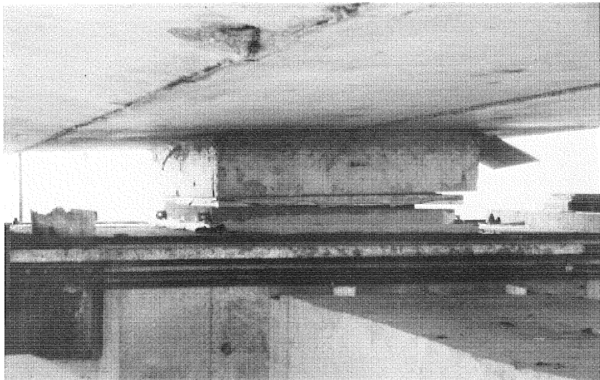
Figure 11. Damaged bearings over east (above) and west (below) columns.
