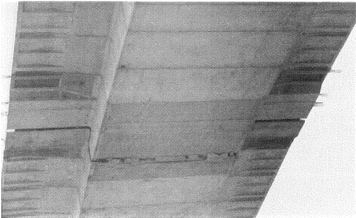
Figure 10. Spalling at the bottom of segments at the damaged joint.
