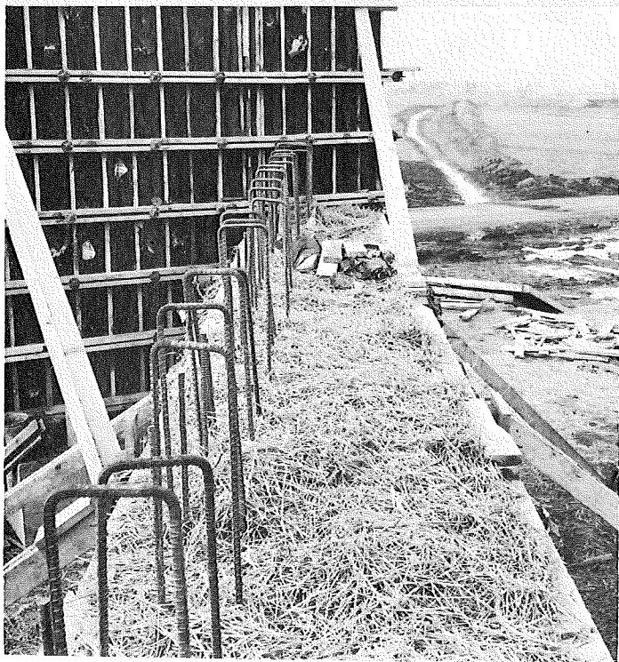
Figure 3 (left). Top of the abutment showing surface covered with straw to retain heat; reinforcement rods project above straw.
