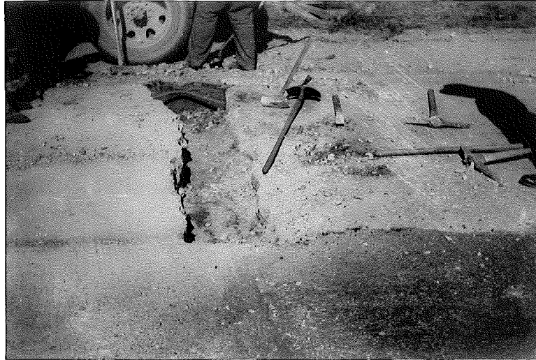
Figure 21. Project 19-3, C5 (1923) US 27 North of Lansing. Blowup in west lane cleaned out ready for filling with bituminous material. No doubt such patches on bituminous capped projects are responsible for certain surface heaves.
