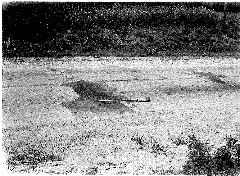
Figure 15. Project 11-3, C3, Benton Harbor East, Blowup No. 9. Note attempt of right slab to ride left slab. Right slab cracked back several feet. Difference in elevation about 2 inches.
