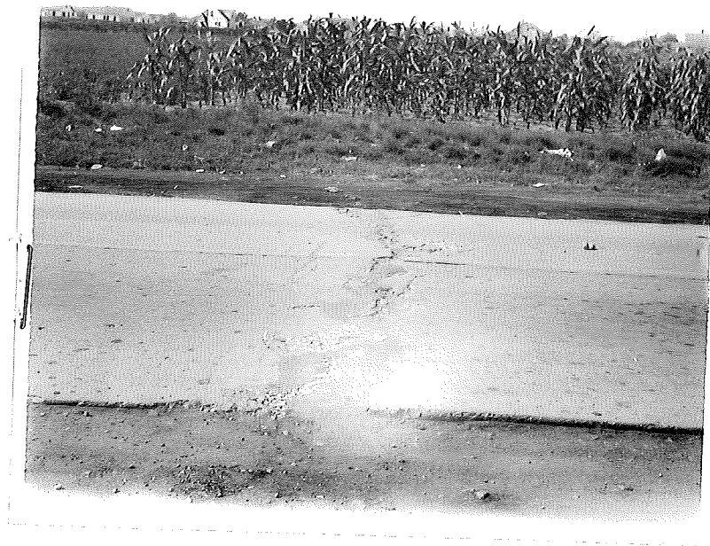
Figure 14. Fresh blowup which had occurred on Project 11-3, C3. Note typical crushing of concrete along crack. Bituminous material indicates that concrete along crack was in advanced stage of disintegration and could not sustain the abnormal compressive forces.
