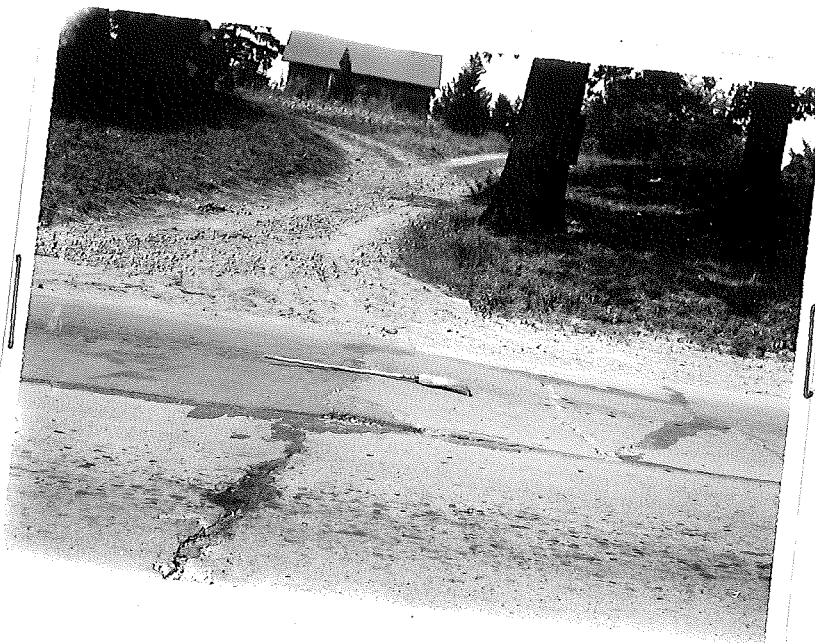
Figure 16. Project 11-3, C3. Blowup No. 10 which was located a short distance from No. 9. In this case note uniform heaving of slabs on each side of crack. Blowup occurred in one lane only.
