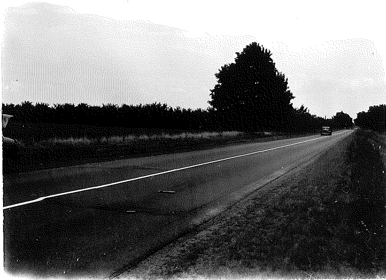
Figure 12. Surface displacement caused by pushing up of concrete slab. Project 78-14, Cl. This was the worse blowup area on project.
