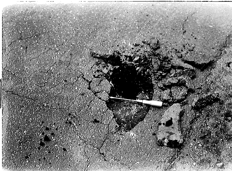
Figure 11. Close view of heave in Figure 10. Note old bituminous patch underneath which under excessive compressive forces has pushed upward causing heaving of the surface course.
