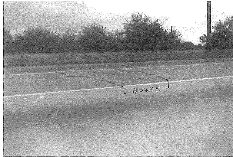
Figure 1. Heaving of bituminous surface center lane, US 16 Howell west, Project 47-14, C 5 & 6
