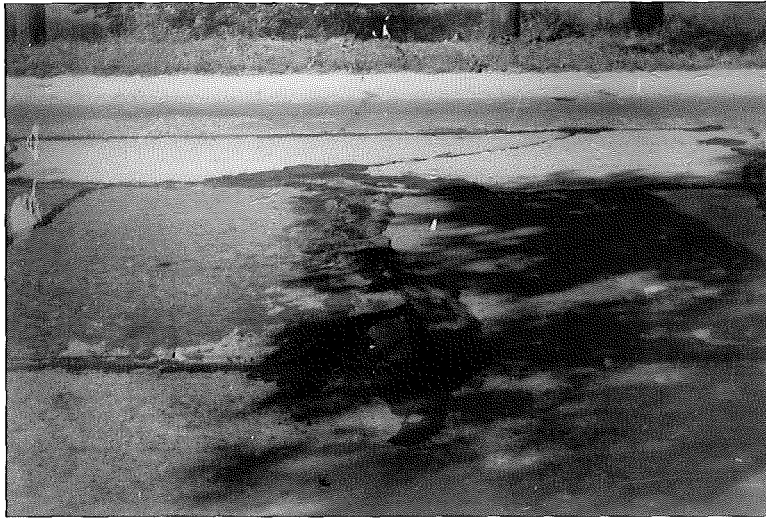
Figure 17. Project 33-24, CE, (1922). Typical blowup area at a crack which has been maintained in service by tar and chips. Such areas are weak points in old pavements and are source of many heaves on bituminous capped projects.
