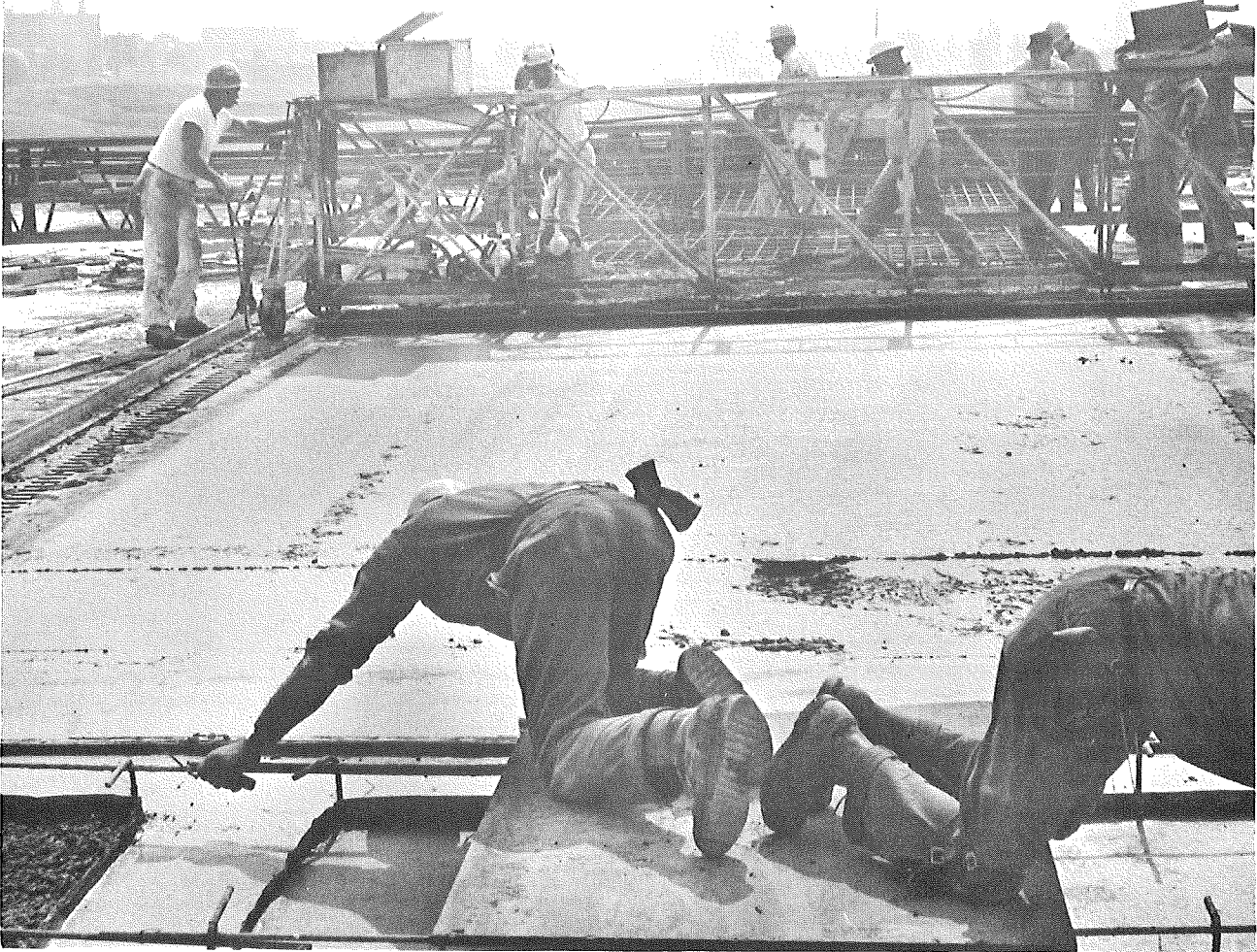
Figure 4 (below). Depressions over the bars visible for four consecutive transverse bars, immediately after passage of finishing equipment.
