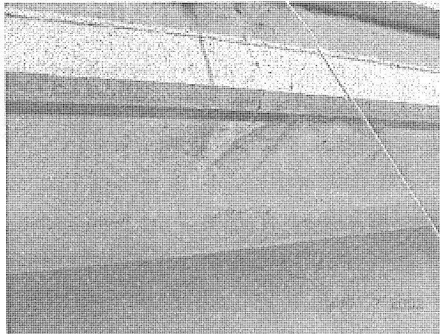
Figure 6-8. Transversal shrinkage cracks at the bottom edge of deck.
