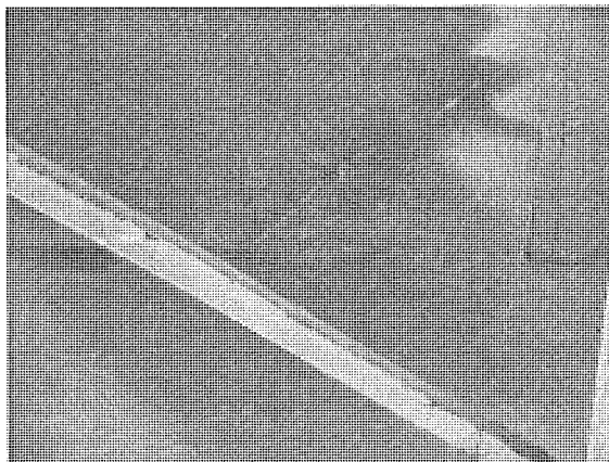
Figure 6-9. Corner shrinkage crack at the bottom of deck.
