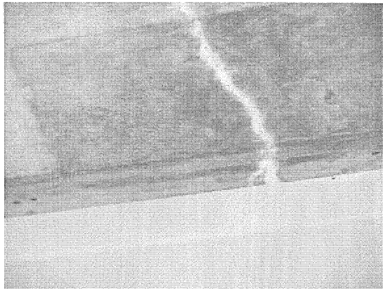
Figure 6-6. Transversal shrinkage crack at the bottom edge of deck.
