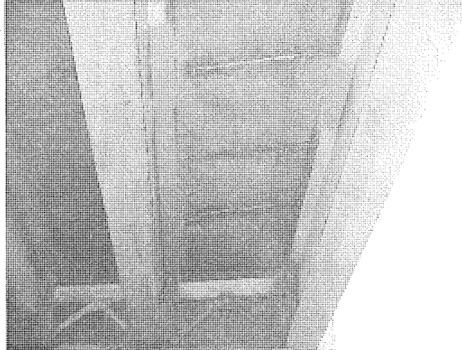
Figure 6-7. Transversal shrinkage cracks at the bottom edge of deck.
