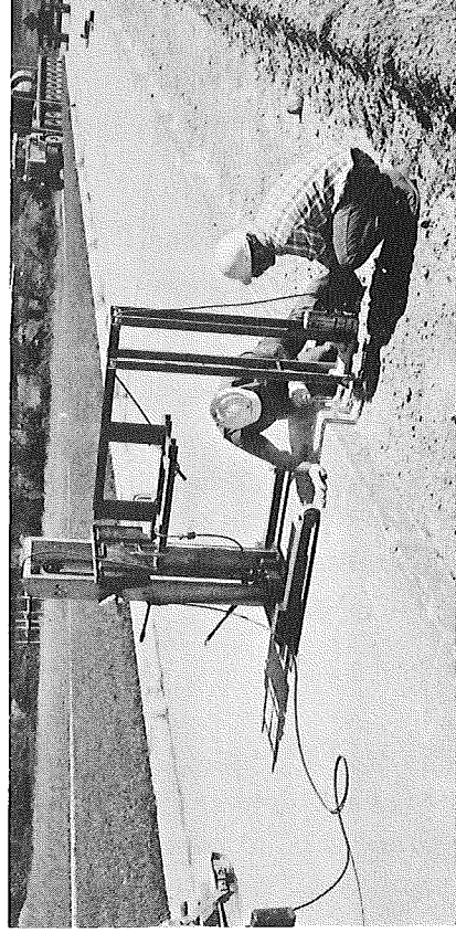
▶ Figure 3. Fixture used to hold roto-hammer in correct alignment while drilling holes.
