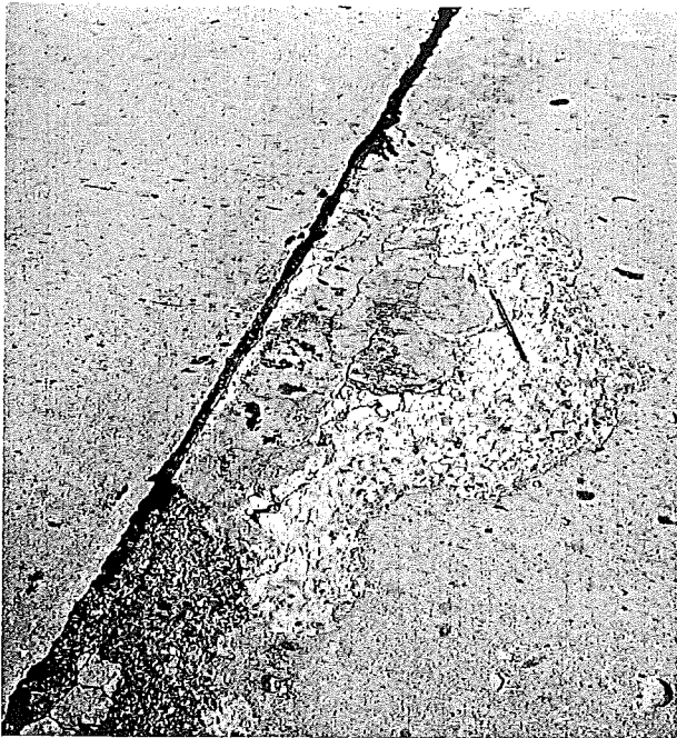
Figure 5. Typical failure indicating possible overfinishing of concrete. Project 47082, C1.
