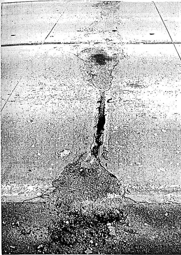
Figure 1. Typical joint condition showing extensive spalling. This joint is to be repaired. Project 47-26, C6.
