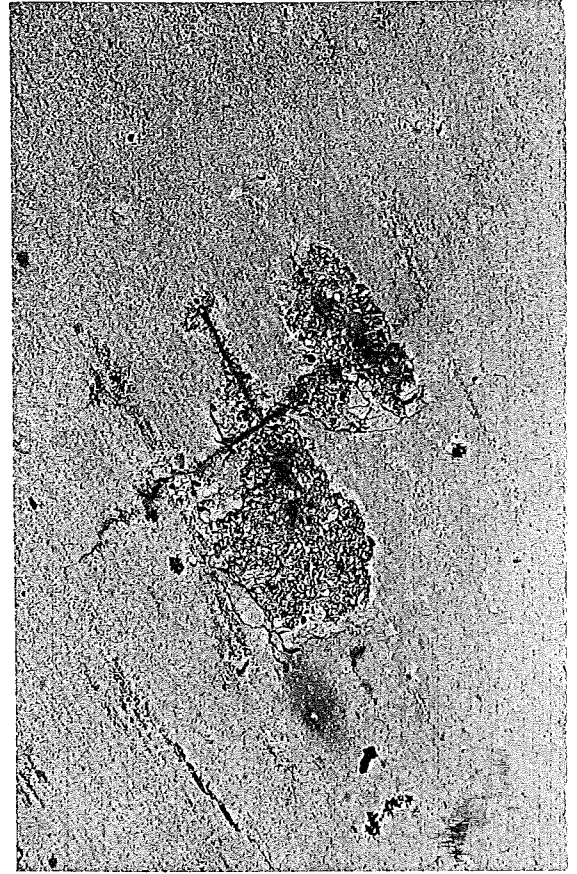
Figure 12. Wire mesh exposed in concrete surface. Project 47-26, C2.
