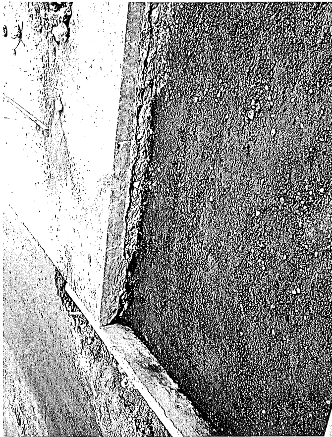
Figure 16. View of damage to remaining pavement caused by breaking out the concrete to be removed. Project 47-26, C6.
