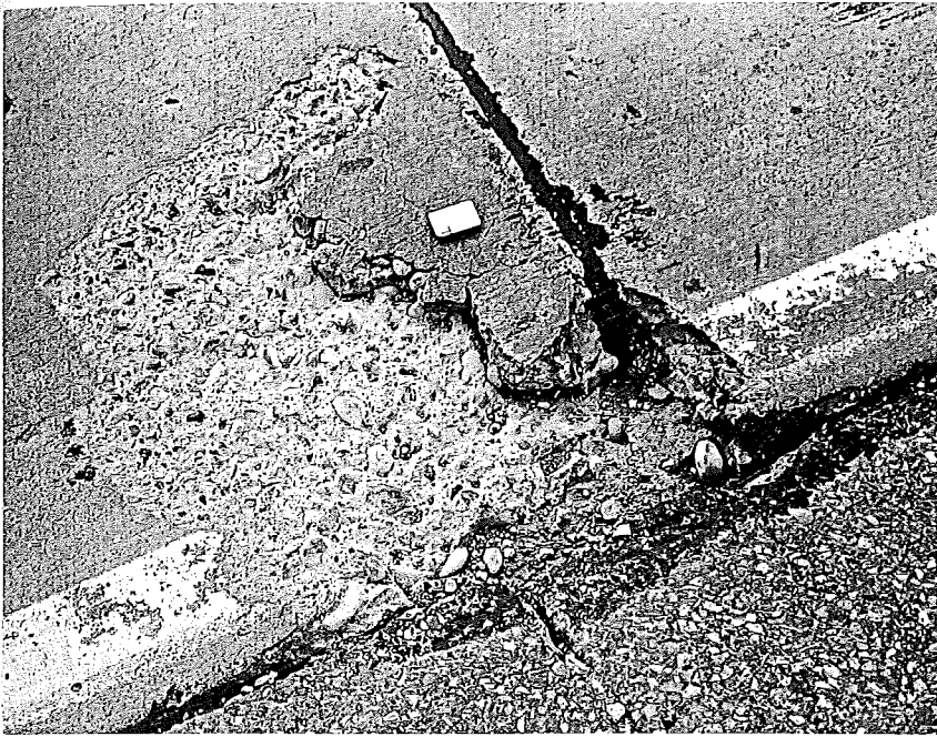
Figure 4. Typical failure indicating possible overfinishing of concrete near joint. Project 47082, C2.
