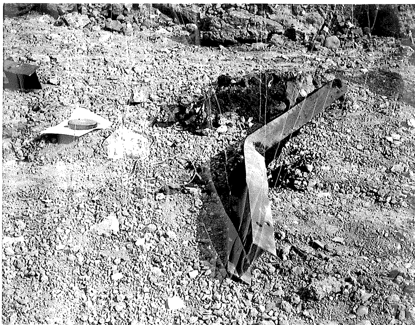
Figure 4. Picture showing typical failure condition of steel post.
