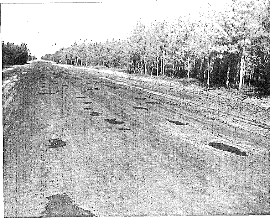
Figure 34. General view RC-2 section, station 144-163. Light area at right is old patch by contractor.
