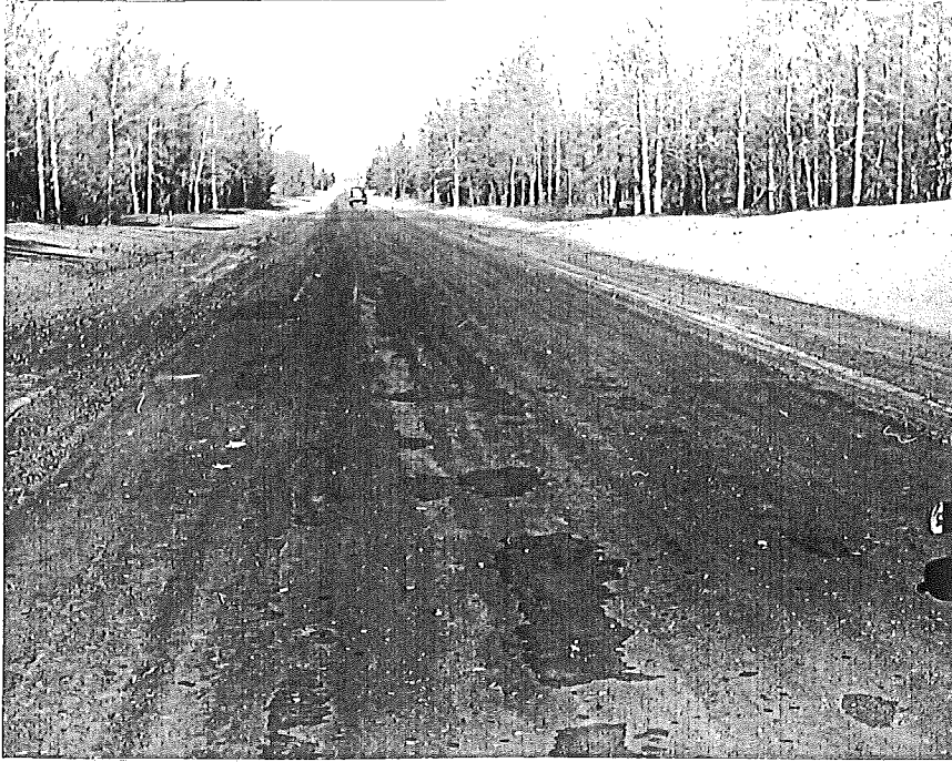
Figure 30. General view of tar section patched throughout length.
