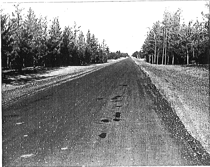
Figure 42. General view MC-2 section, station 246. Surface poor, rutting.
