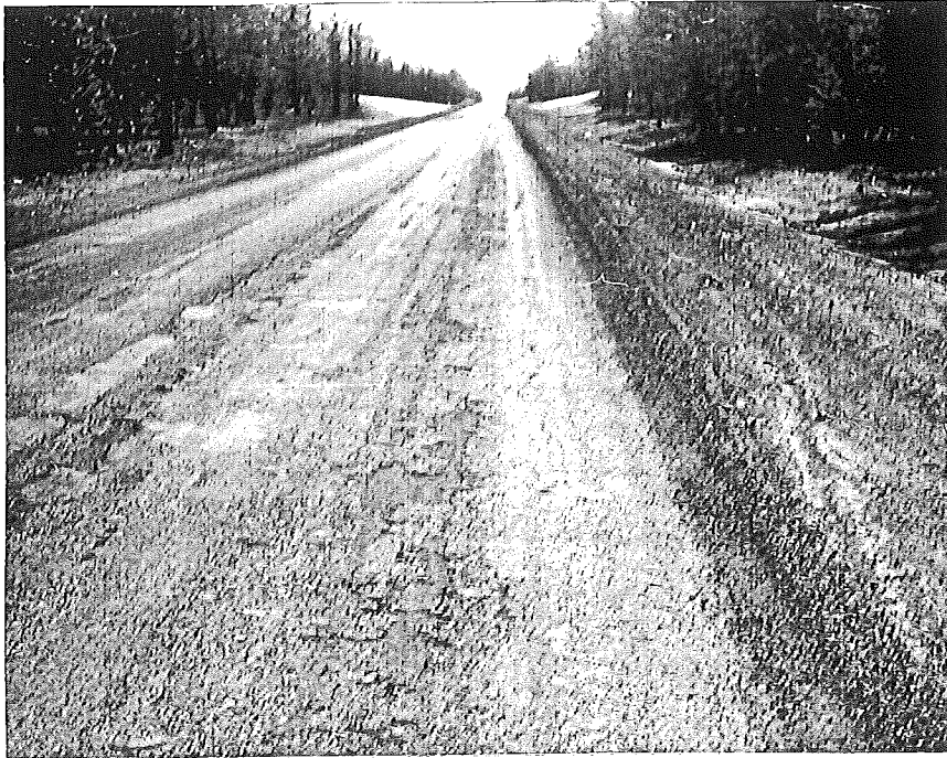
Figure 28. General view AE-7 section with surface treatment. Note stripping of surface from base.
