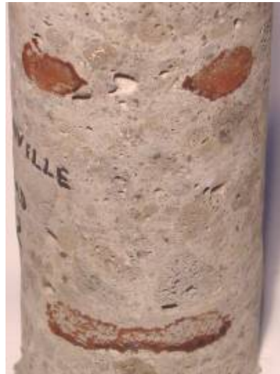
Figure 3.36. Core 2b rust in the reinforcement bars
