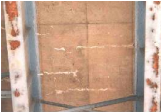
a. Transverse cracks and white traces
