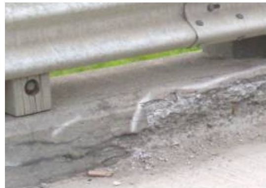
b. Deteriorated section and white traces
