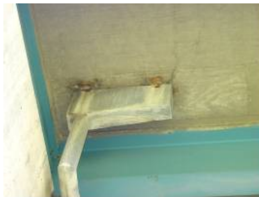
e. Rust traces from reinforcement around the drainage holes
