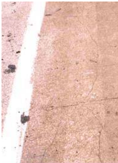
Figure 3.142. Cracks at the top surface
