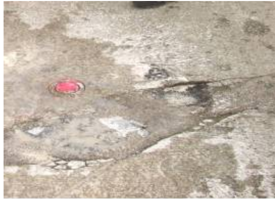
Figure 3.128. Deterioration in the joint
