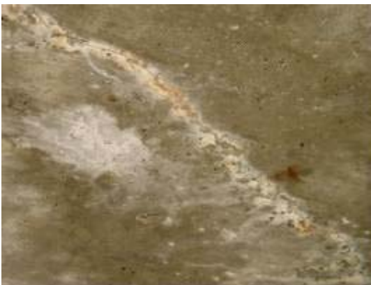
Figure 3.27. White traces on the bottom surface
