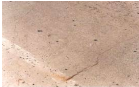
b. Transverse cracks with rust traces
