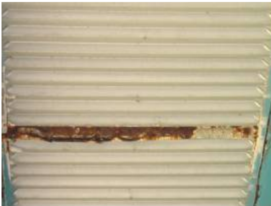
b. Corrosion in the SIPMF oriented transversely
