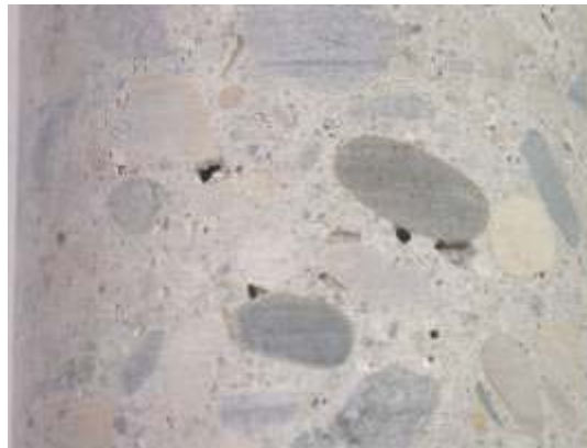
Figure 3.108. Core 6e many locations of entrapped air
