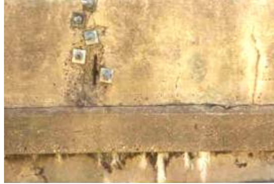
Figure 3.145. White traces and rust traces at Cracks
