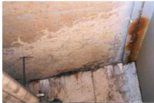
b. Cracks and rust traces
