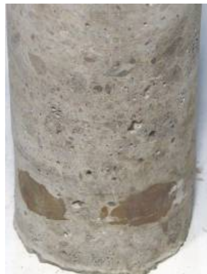
Figure 3.58. Core 3b voids and rust in the reinforcement
