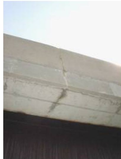
Figure 3.164. Cracks with white traces propagated in the parapet and the whole depth of the slab
