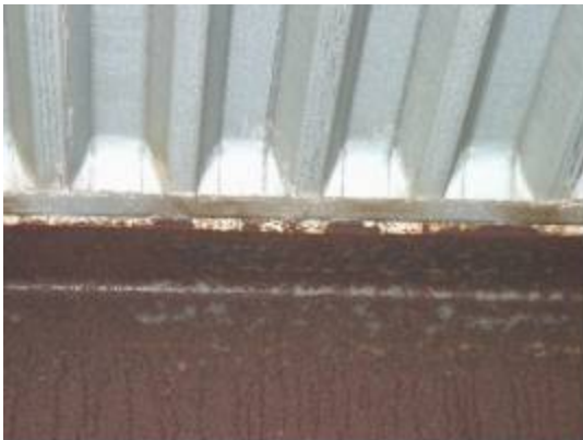
Figure 3.169. White and corrosion traces at the connection between steel beams and the SIPMF
