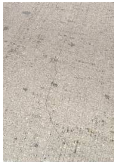
b. Diagonal and transverse cracks
