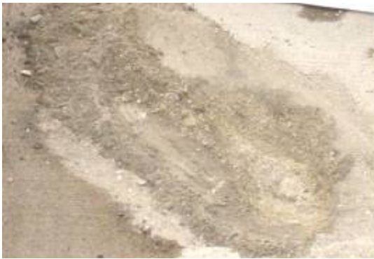
a. Large depression in bridge deck
