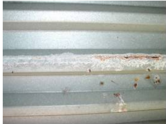
b. White and rust traces
