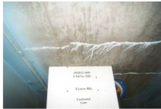
b. White traces with transverse crack
