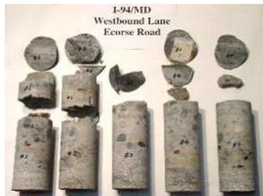
Figure 3.146. The 5 cores taken from Bridge Deck Number 9 (Structure No. S10-82022)
