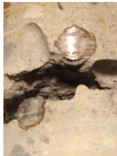
b. Rust in the reinforcing steel
