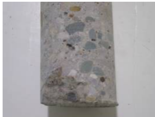
Figure 3.11. Core 1a shows large region of honeycombing
