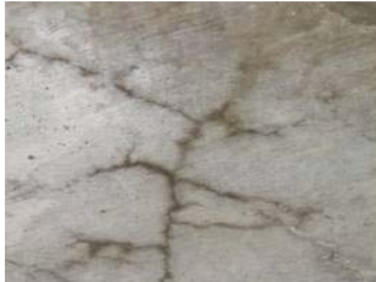
b. Diagonal and Transverse cracks
