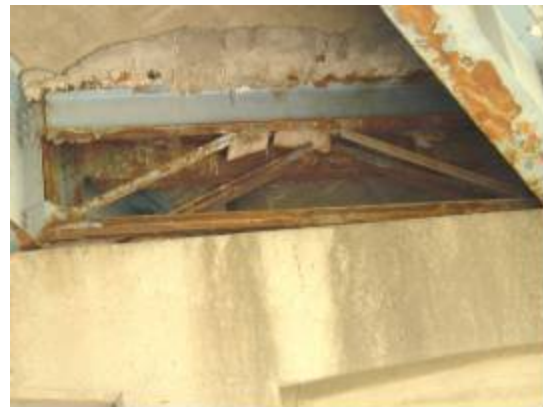
b. Rust traces
