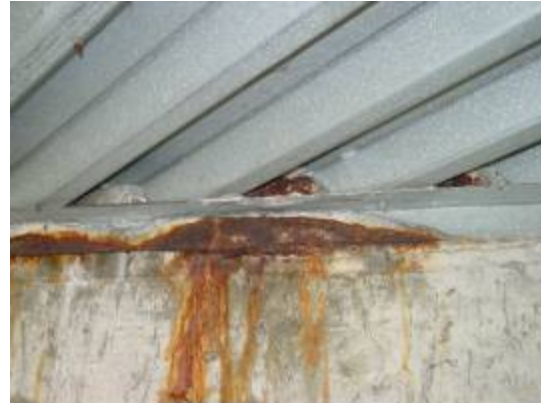
Figure 3.170. White and corrosion traces at the connection between SIPMF and the abutment
