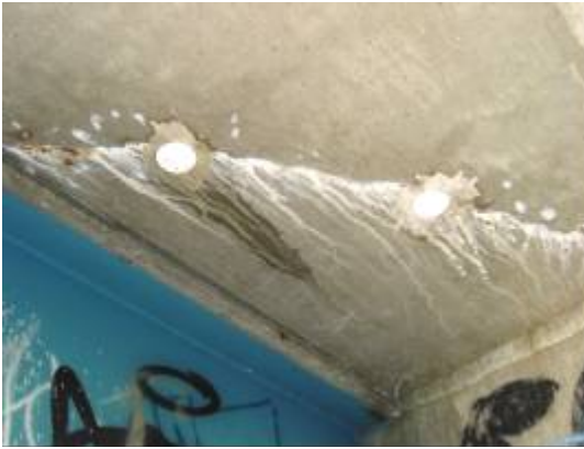
a. Diagonal cracks with white traces
