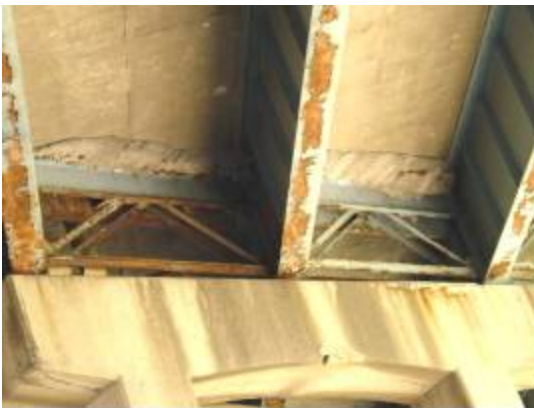
a. Deteriorated concrete cover
