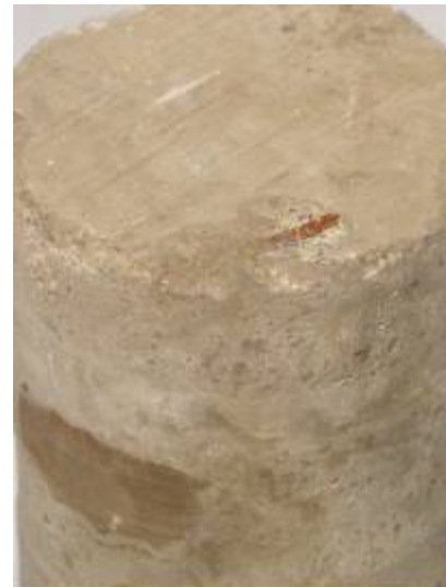
Figure 3.66. Pop-out in concrete Core 3e
