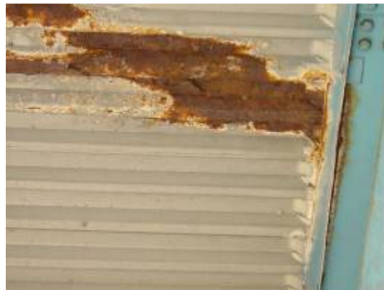
c. Corrosion in SIPMF and steel beam at the connection
