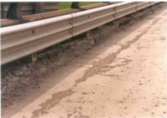
a. Severe deterioration along the curb
