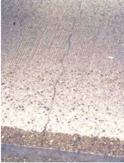
Figure 3.161. Top cracks propagated transversely in the slab
