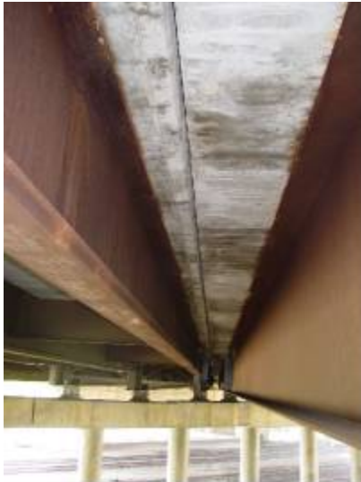
Figure 3.167. Corrosion and white traces on the bottom face of the cantilever slabs
