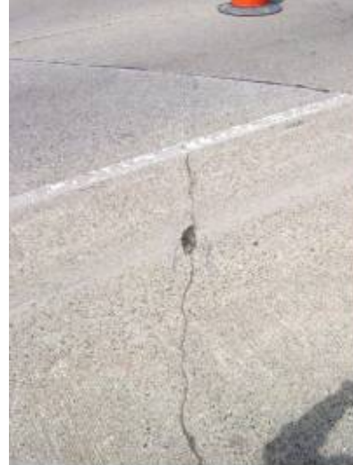
Figure 3.162. Top cracks propagated diagonally in the slab
