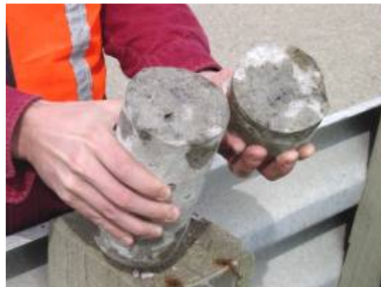
Figure 3.38. Presence of horizontal crack in Core 2c
