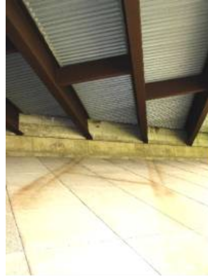
Figure 3.168. Corrosion traces underneath the steel beams
