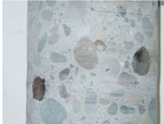
Figure 3.175. Core 10a small voids in the concrete
