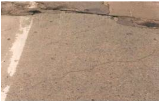
a. Diagonal cracks
