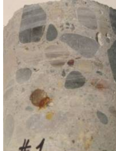
Figure 3.148. Core 9a rust in the reinforcement bar
