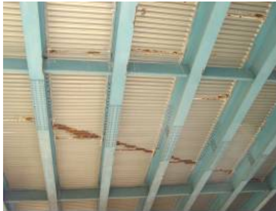
a. Corrosion in the SIPMF oriented diagonally
