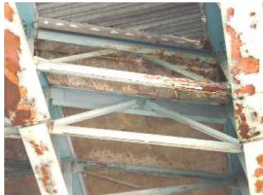
Figure 3.130. Rust in the connection between steel girders and SIPMFs
