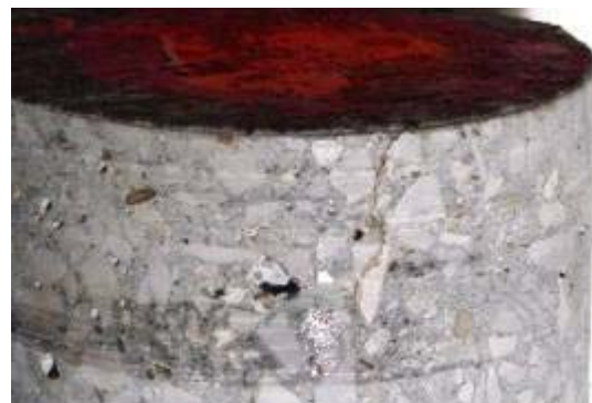
Figure 3.156. Core 9e hairline cracks at the top surface layer of the deck
