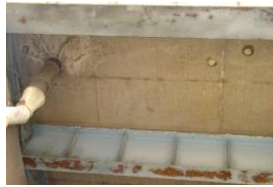
d. White traces around drainage opening
