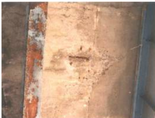
a. Deteriorated concrete cover and rust traces
