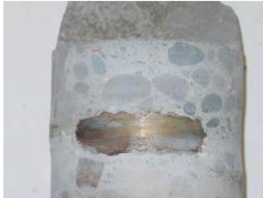
b. Reinforcement bar had traces of corrosion
