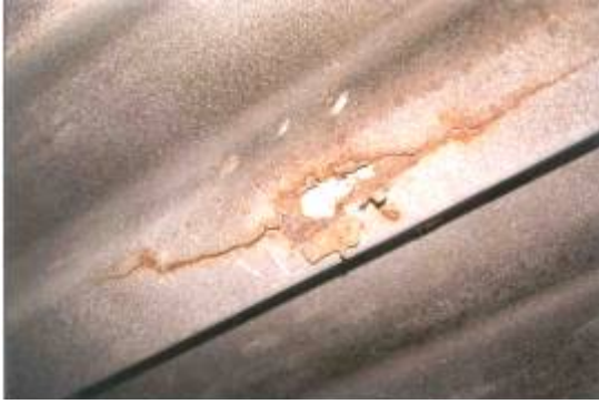
Figure 3.144. Excessive corrosion in SIPMF
