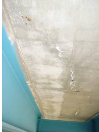
b. Longitudinal cracks with white traces
