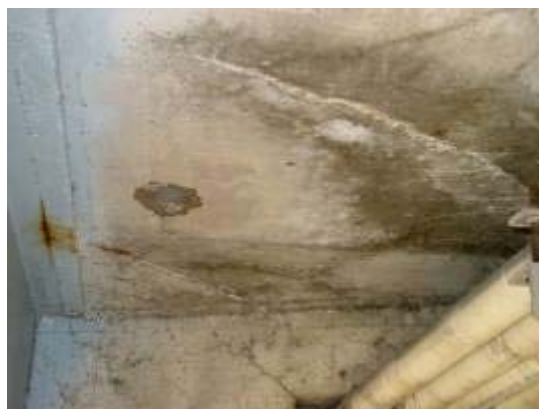
Figure 3.28. Rust traces on the bottom surface
