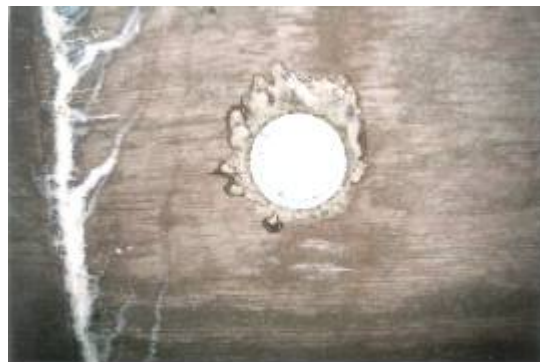
Figure 3.84. White traces near coring location
