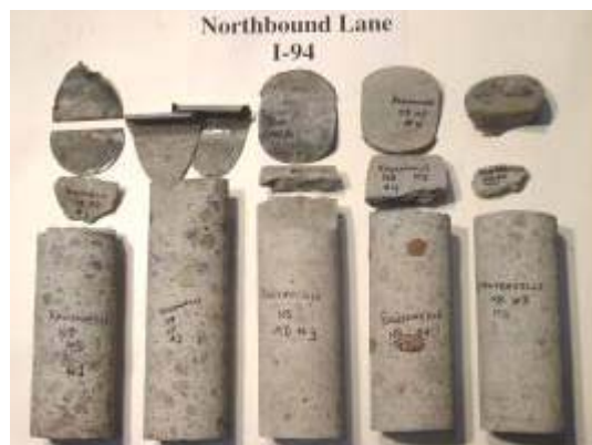
Figure 3.116. The 5 cores that were taken from Bridge Deck Number 7 (Structure No. S03-81041)
