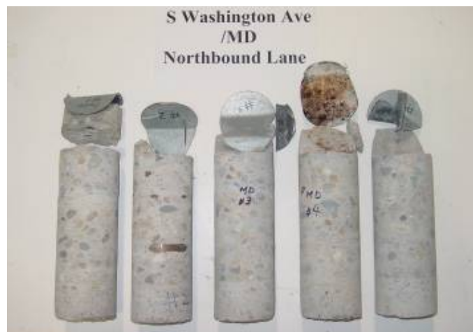
Figure 3.102. The 5 cores that were taken from Bridge Deck Number 6 (Structure No. R01-13012)
