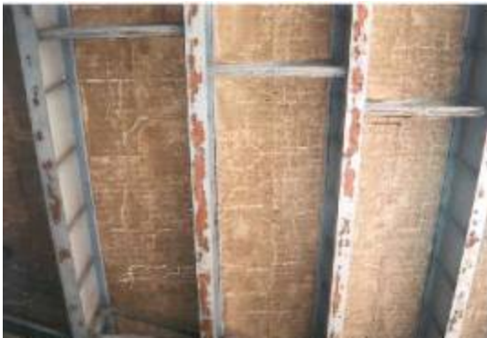
c. Cracks and white traces (small rectangles)
