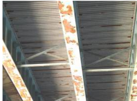
b. General view of the rusted SIPMFs
