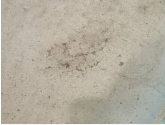
Figure 3.29. Honeycombing at the bottom surface of the slab
