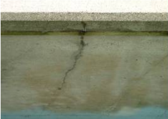
Figure 3.24. Cracks through the slab thickness
