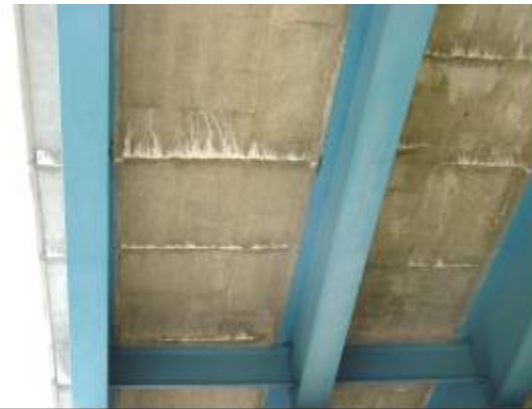
c. Transverse cracks with white traces
