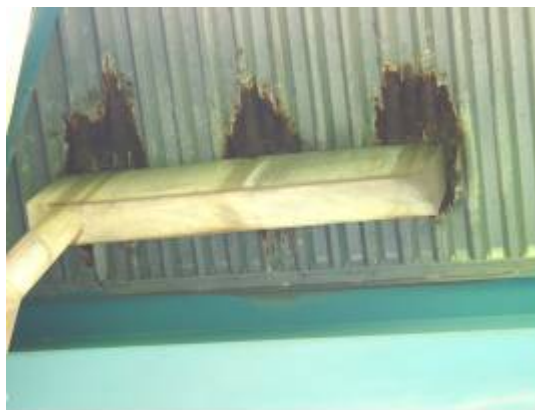
Figure 3.101. Corrosion around the hole in the deck with SIPMF
