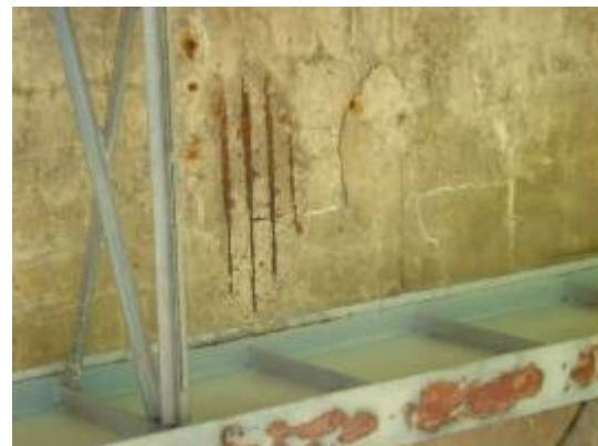
b. Reinforcement bars rusted
