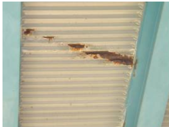
c. Corrosion and white traces in the SIPMF
