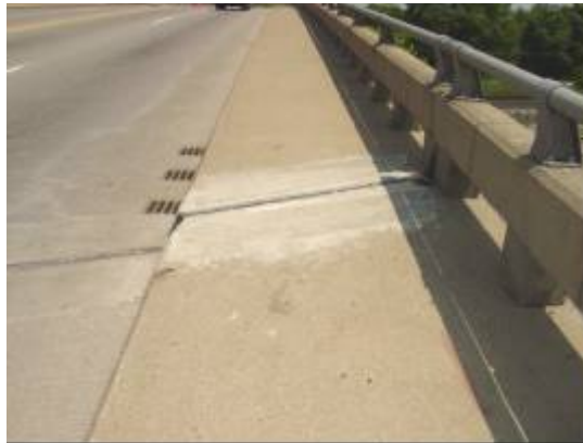
Figure 3.98. Different types of concrete around the joints
