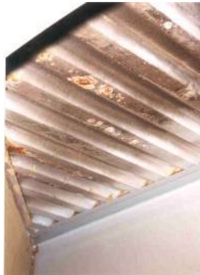
Figure 3.143. Traces of corrosion in SIPMF
