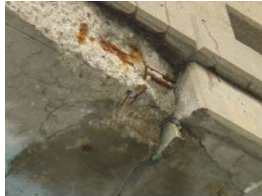
Figure 3.30. Deterioration of the concrete cover and rust traces at the joint
