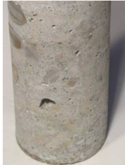
Figure 3.133. Core 8a honeycombing and large single void in the concrete
