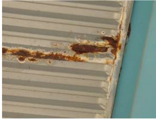
a. Corrosion and white traces near the connection
