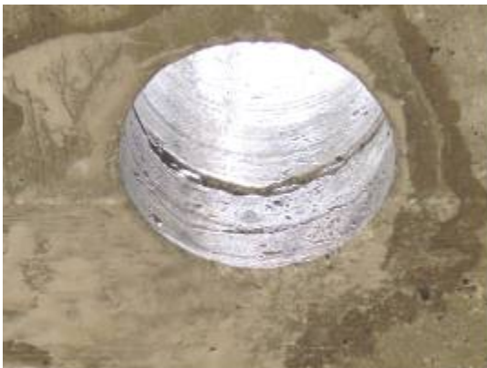
Figure 3.37. Crack in the thickness of the slab (Core 2c location)
