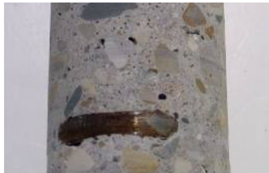
Figure 3.104. Core 6b many honeycombing and rust in the reinforcement bars
