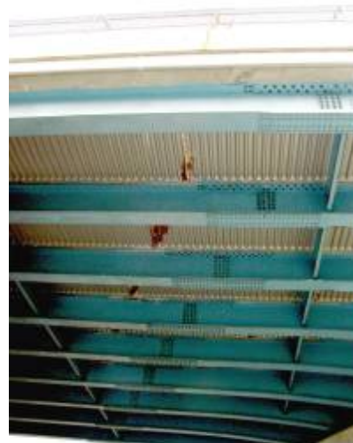
Figure 3.97. Corrosion at the SIPMF
