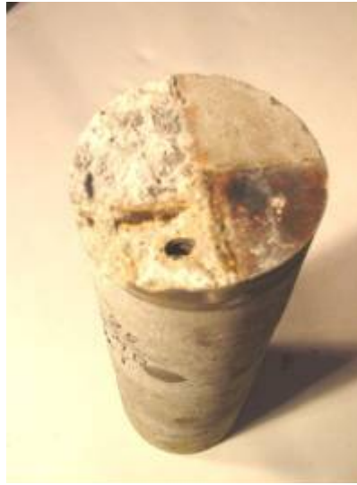
b. Large void and rust at the bottom
