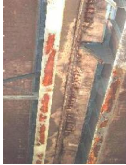
b. Rust and white traces
