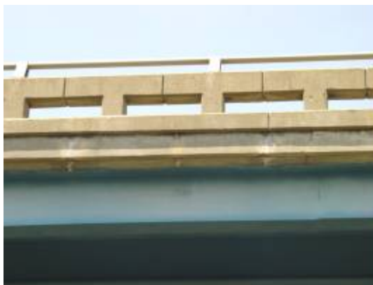
Figure 3.7. Cracks propagated through the sides
