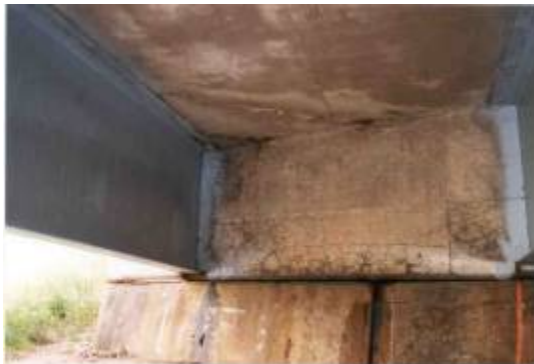
a. Water leakage
