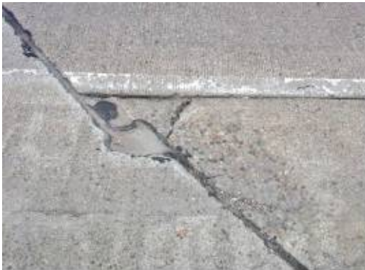
Figure 3.163. Top cracks propagated around the joint
