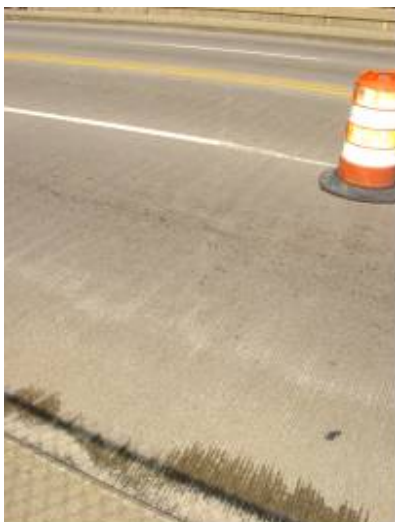
Figure 3.96. Cracks propagated on the top surface of the deck slab
