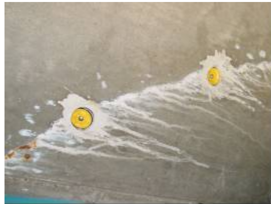
d. Cracks with corrosion and white traces in the direction of slope
