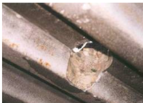
e. Resulting hole in a concrete deck slab with SIPMF, view from below
