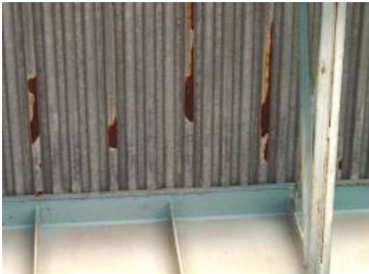
a. Rust traces in SIPMF
