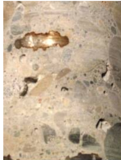
Figure 3.151. Core 9c Large voids and rust in the reinforcing steel
