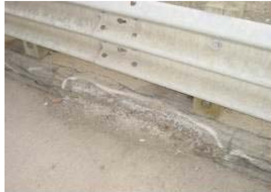
Figure 3.25. Severe deterioration of the curb
