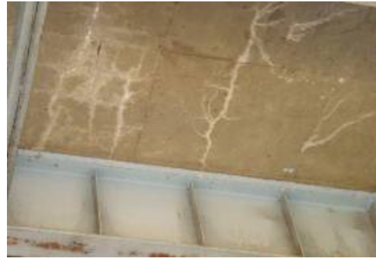
b. Transverse and longitudinal cracks
