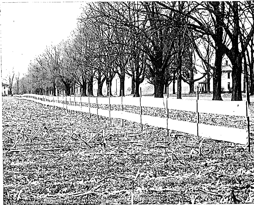
Figure 34. Long stretch of 2-panel fence on west side of M-40 between Dowagiac and Decatur. Van Buren County, 2-7-52
