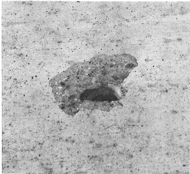
A popout with clear breakaway of overlying mortar due to pressure associated with heating effects just below the surface (popout: 3-1/2 in. diam).
