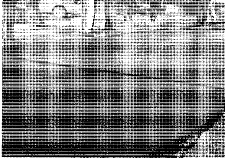
Figure 7. Transverse fault in Gussasphalt caused by settlement on screed when paver stopped moving.
