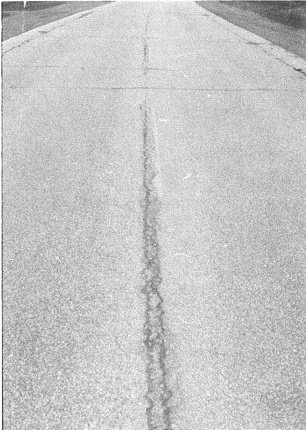
◀ Figure 3. Low-Severity Longitudinal Joint Reflection Cracking.
