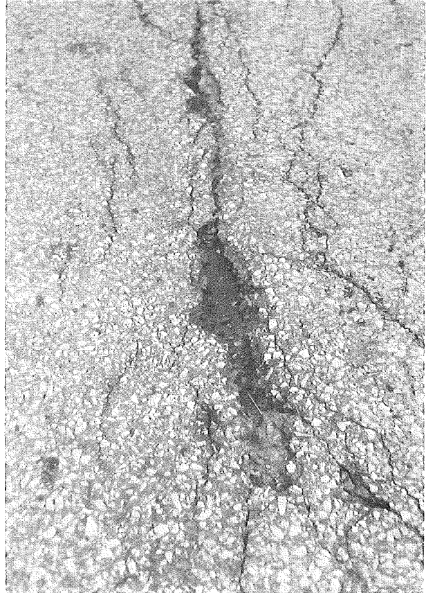
▲ Figure 4. Medium Severity Longitudinal Joint Reflection Cracking.
