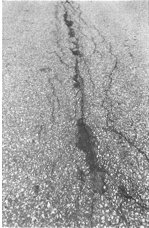
▲ Figure A2. Medium Severity Longitudinal Joint Reflection Cracking.
