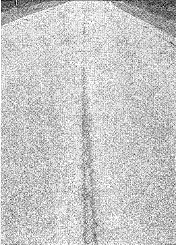
◀ Figure A1. Low-Severity Longitudinal Joint Reflection Cracking.
