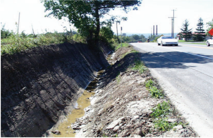
Deep ditches such as this are a safety hazard.
