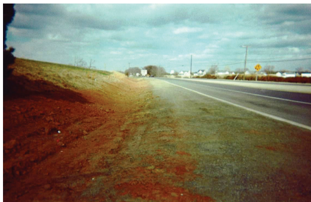
This ditch was reshaped to provide a safe recovery area for errant vehicles.
