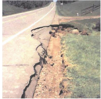
Deterioration of pavement edge and shoulder due to poor drainage.
