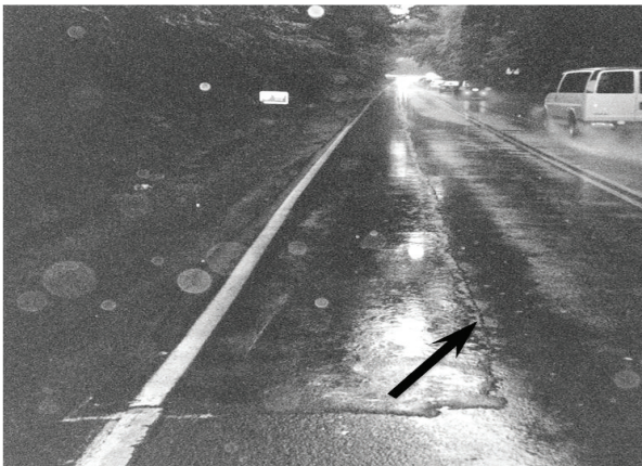
The edge of this partial pavement overlay is causing water to be retained on the travel way surface.
