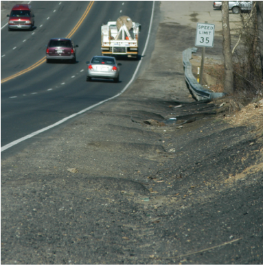
A traversable drainage ditch such as this provides space for vehicle recovery.
