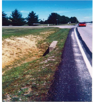
This culvert headwall is a roadside hazard.
