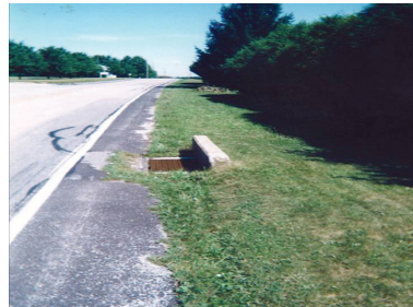
The headwall is sticking up almost a foot in a relatively flat recoverable area. It can snag a vehicle and bring it to an abrupt stop or cause it to overturn.
