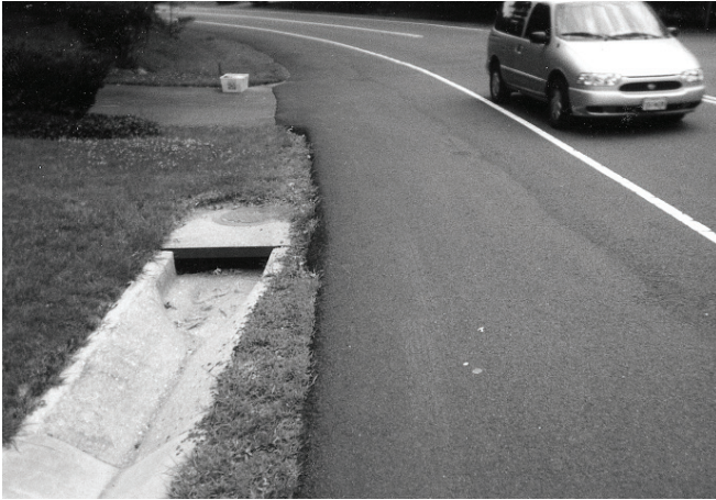
This culvert has a rather large opening which could cause a vehicle that hits it to go out of control.
