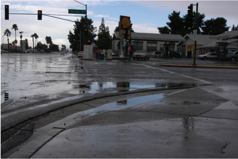
Water standing in the roadway.
