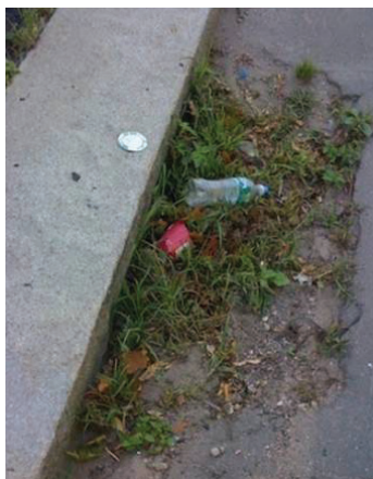
A clogged drain can easily be detected during a field survey.
