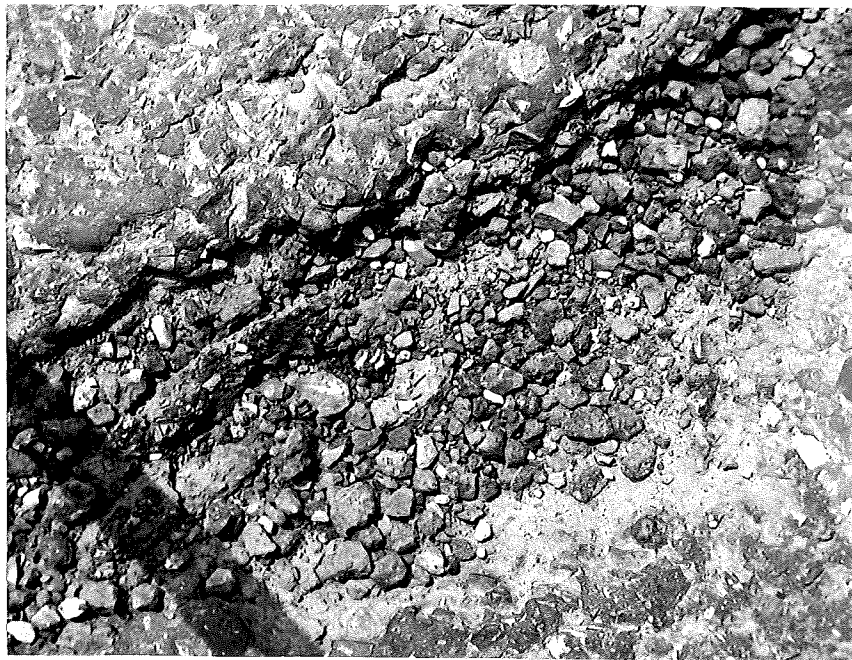
B. Close-up of a section of above joint showing destruction of bituminous surface by extruded filler.
