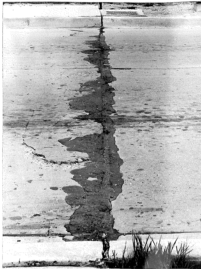
A. Expansion joint in south approach to Main St. Bridge, Lansing; Project U 33-66, Cl. Note extrusion and breakdown of filler.
