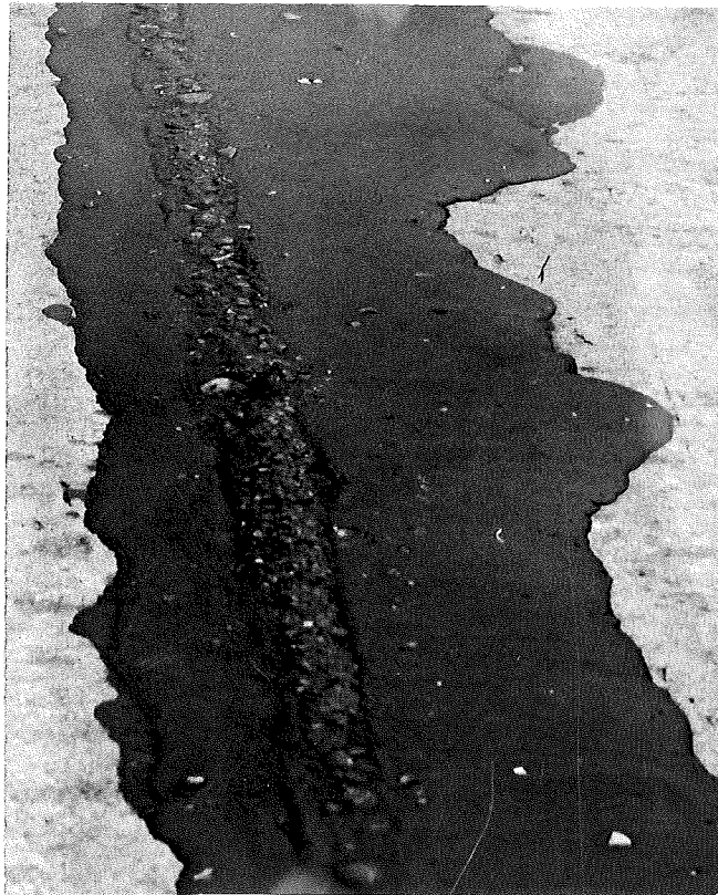
B. Close-up of joint at Station 633+20, Southbound lane, to show extrusion and displacement of joint material.
