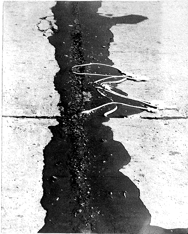
A. Joint in southbound lane, Station 637+20.
