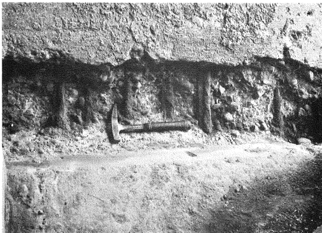
Figure 11. Overall and close-up views of spalled area at base of west fascia rib at north abutment.
