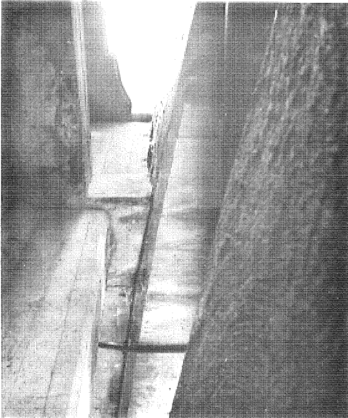
Figure 2 (above). View of header wall of west fascia rib at north end of Span 3. Note weep holes through header and salt stains down inside face of rib caused by drainage from deck construction joint.
