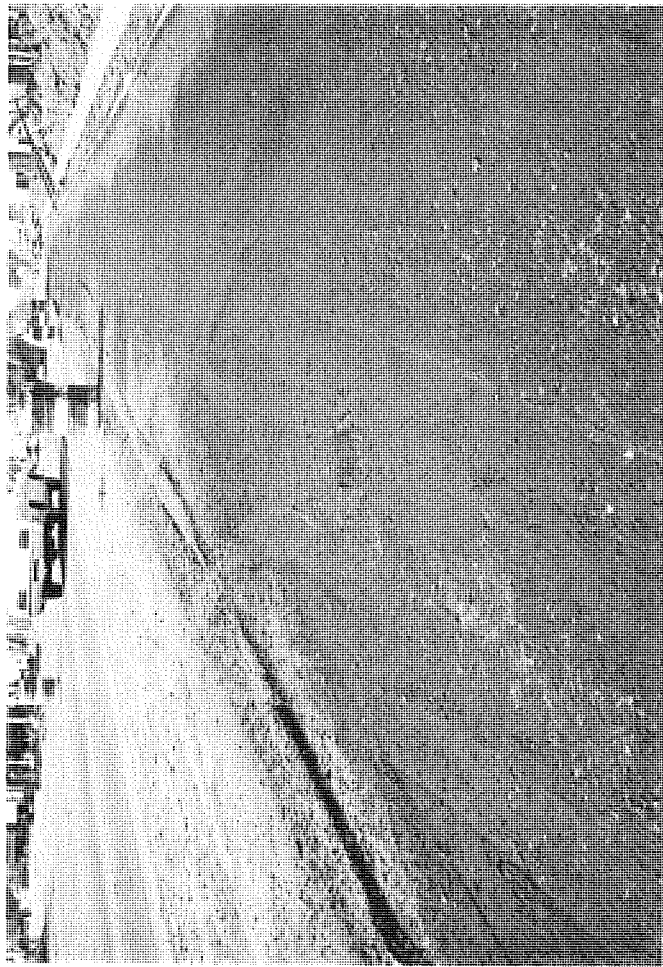
Figure 4. Moist appearance of the compacted cold-mix base material. Drying, generally progressing inward from the edges is accompanied by increased stability.
