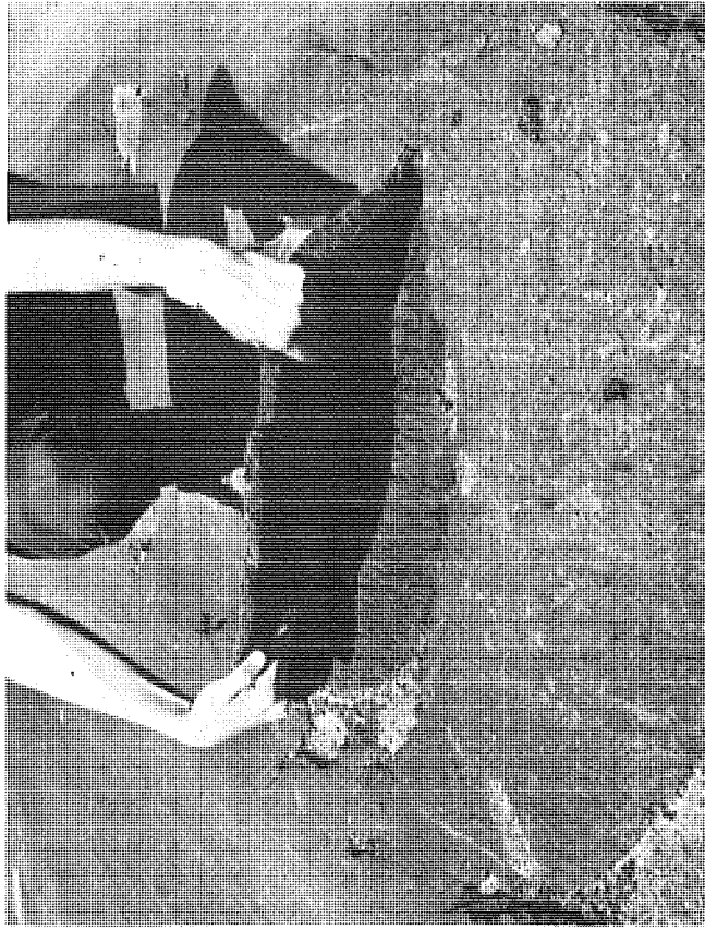
Leveling course separating from emulsion black base.
