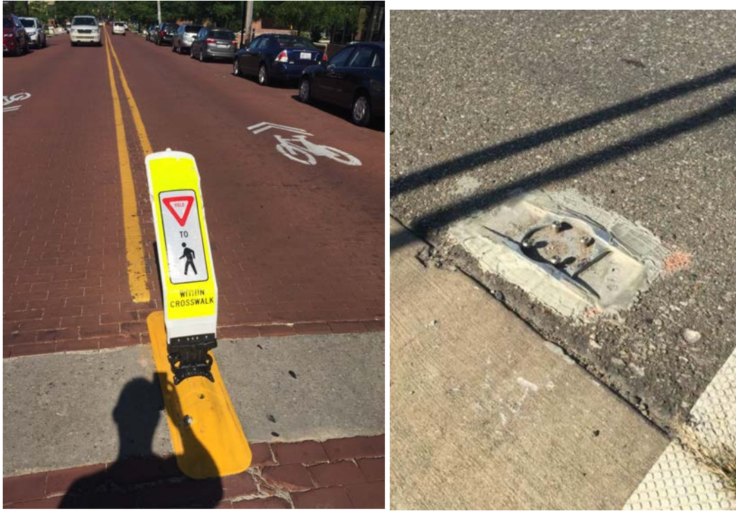
Figures 5.2-a. (above left) shows an R1-6 sign installed on a removable curb base that was damaged during the study. Figure 5.2-b (above right) shows a sheared base of a flush mounted sign.
