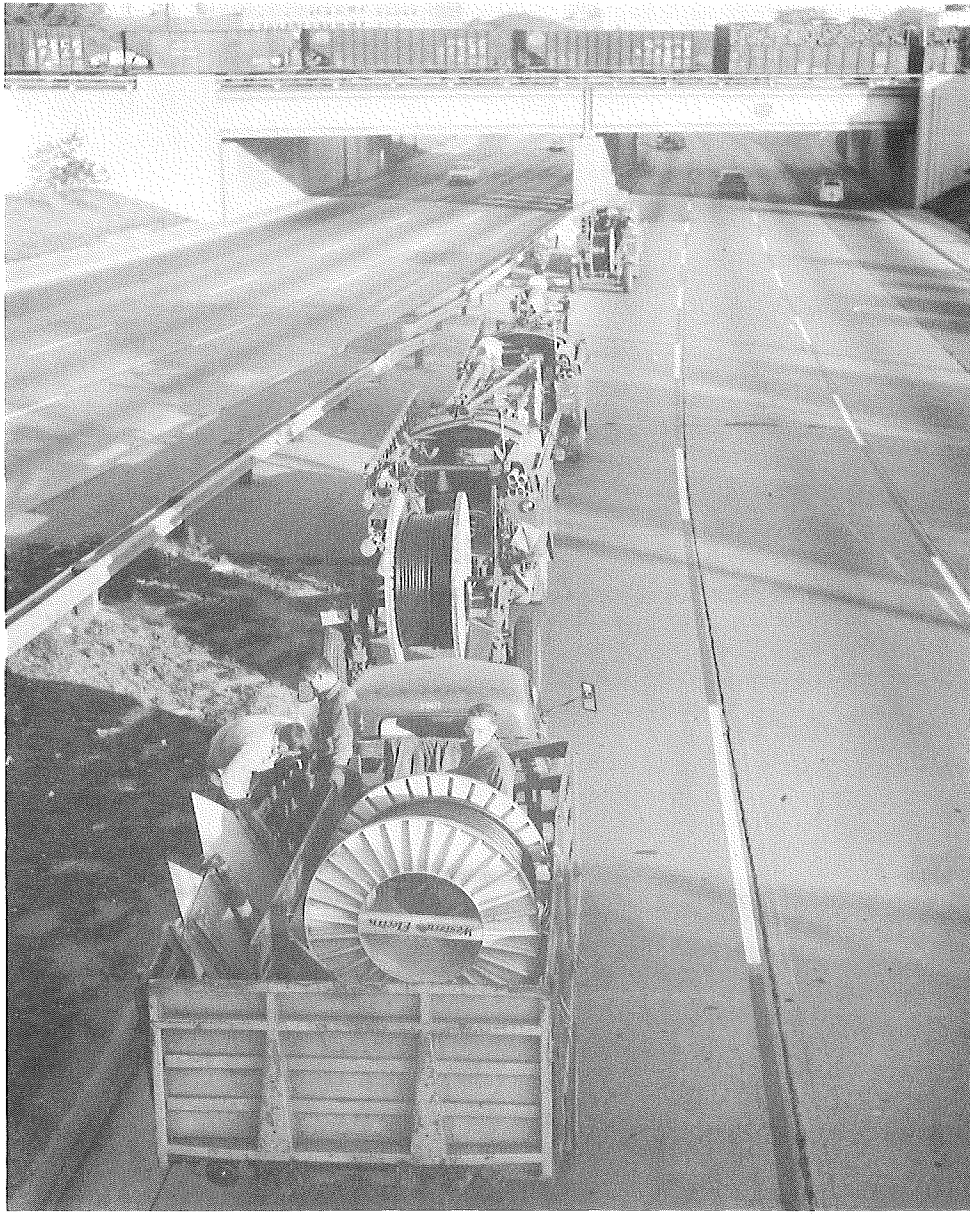
Michigan Bell Telephone Crews Entering Freeway and Preparing to Lay Cable for the Television Surveillance Project.
