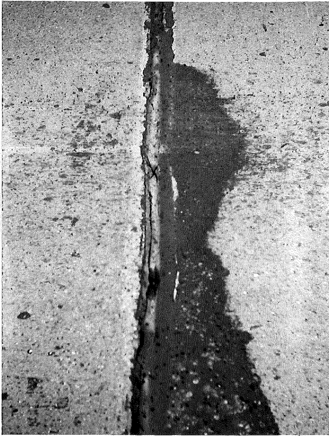
A. Station 645+50 N. Failures in Both Cohesion and Adhesion.
