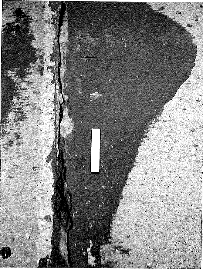
A. Station 655+50 N. Failures in Both Adhesion and Cohesion.
