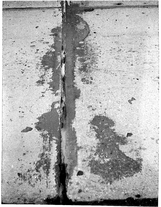
B. Station 646+45 S. Failure not as Extreme as at Left.
