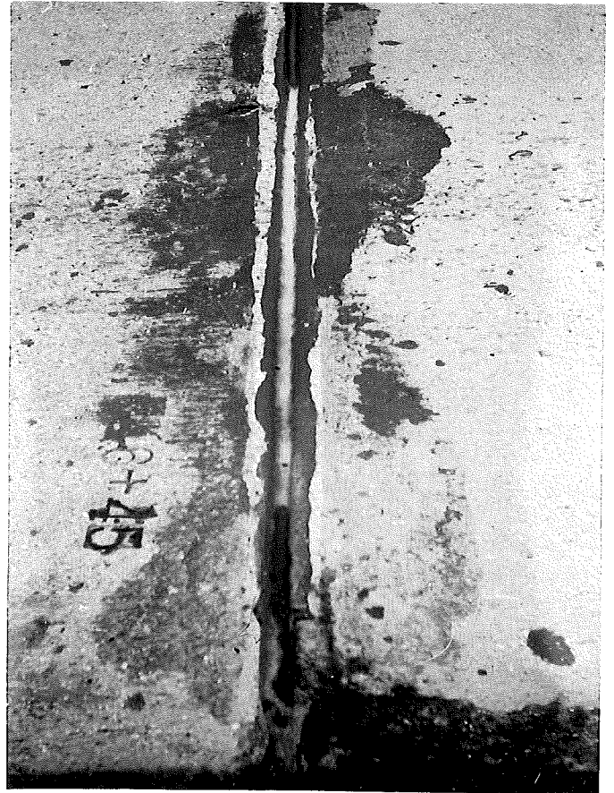
B. Station 646+45 N. Adhesion and Cohesion Good. Slight Resinification of Sealer Surface.
