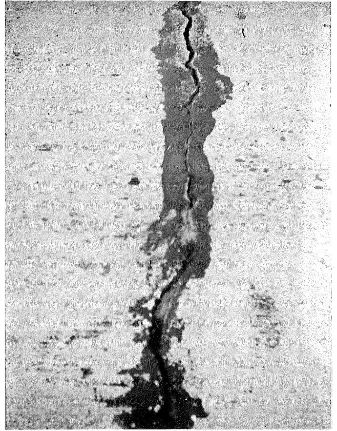
B. Station 582+60 N. Sealed with Brand C. Failure in Cohesion.
