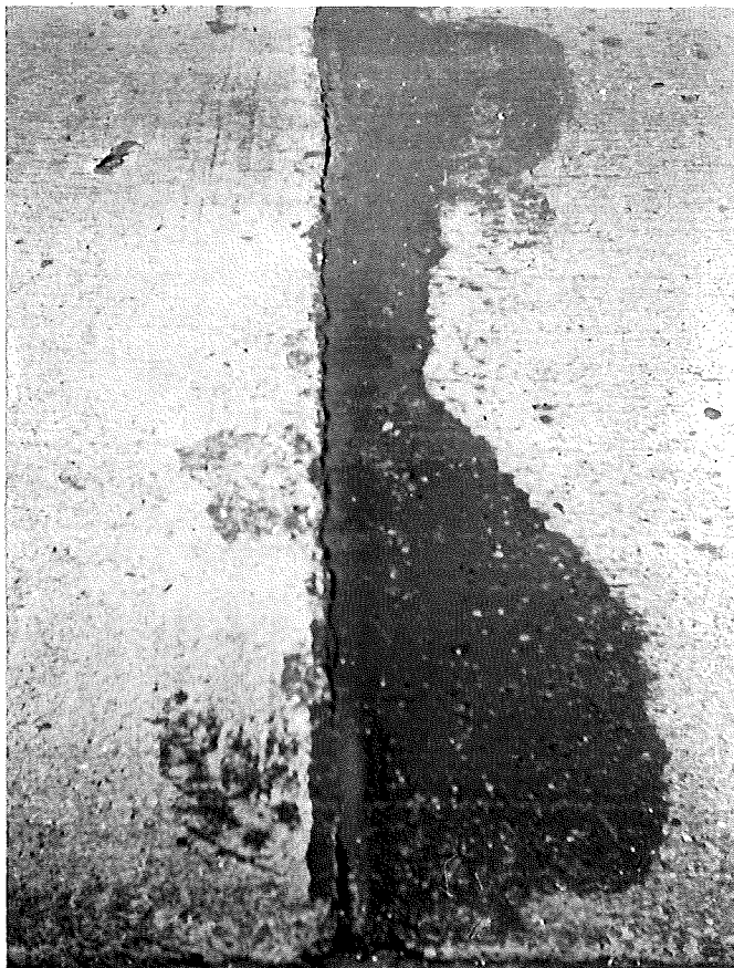
A. Station 514+97 S. Adhesion to One Joint Face Lost.
