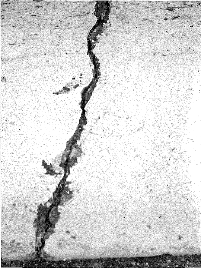
A. Station 582+60 S. Sealed with Brand A. Failure in Cohesion.
