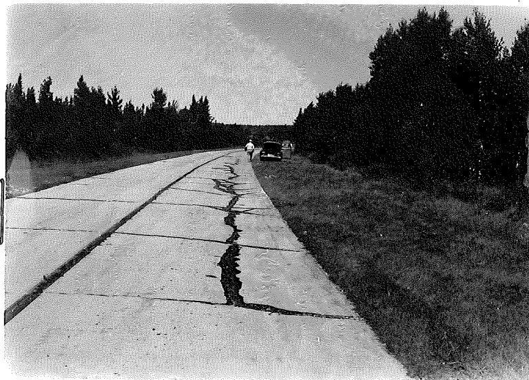
Figure 4. 49-7, C1. General view of cracking at Station 222+00. Looking north. Slabs settled along longitudinal crack, however, slabs have not faulted. Crack about 1/2 inch wide at top.
