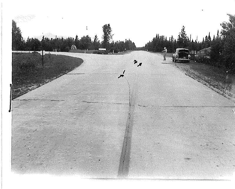
Figure 15. 49-7, C1, General view of wye looking north at Station 422+00. Note unusual construction procedure at wye emphasized by curved cracks joining the center line of US 2 with center line of County Road (1). Also note similar curved crack joining the right edge of the slab on US 2 with that on County Road (2)
