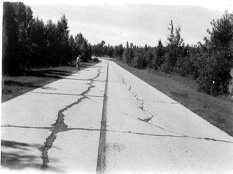
Figure 2. 49-7, C1, General view of cracking at Station 211+00 to 212+50. looking south. Heaving occurred at crack on right, settlement at crack on left. Note how snow plows have scraped crack on right.
