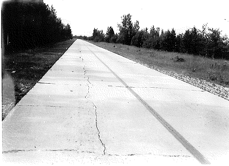
Figure 13. 49-7, C1, View of cracking looking south from Station 414+00. Slab constructed on cut and fill section.
