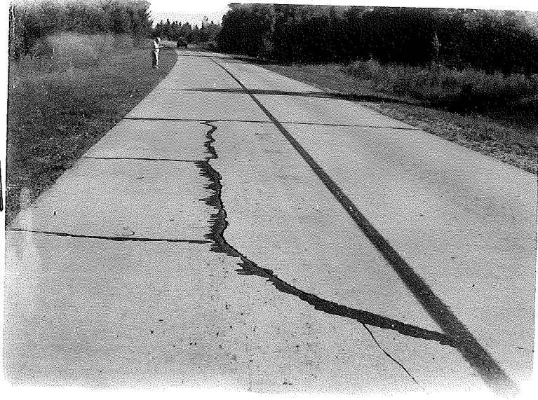
Figure 9. 49-7, CI, Cracking at Station 347+50, looking south.
