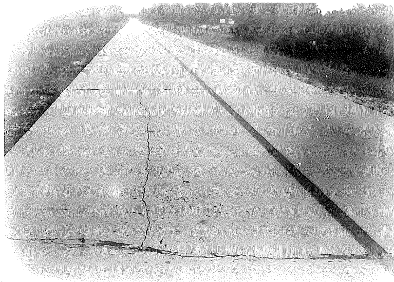
Figure 12. 49-7, C1, View at Station 383+00, looking south. Pavement on cut and fill section. Cracks need sealing.
