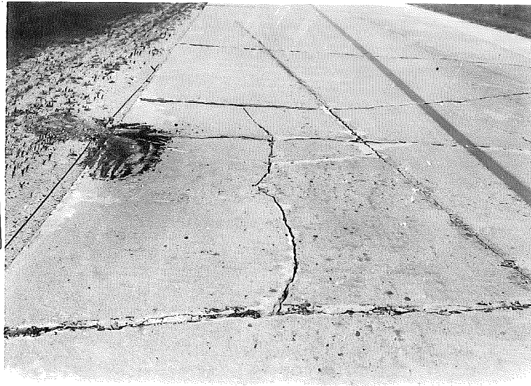
Figure 14. 49-7, C1, View at Station 422+10 looking south showing bad break up in this area. Note soundness of concrete adjacent to cracks.
