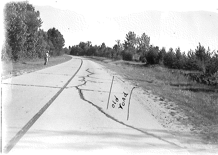
Figure 10. 49-7, CI, Cracking at Station 553+00, looking south. Note that this area is where old road joins new pavement.
