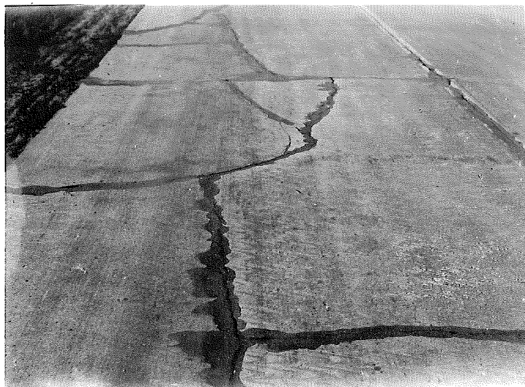
Figure 6. Typical condition of cracked areas. Station 232+00 looking south. Project 49-7, C1.
