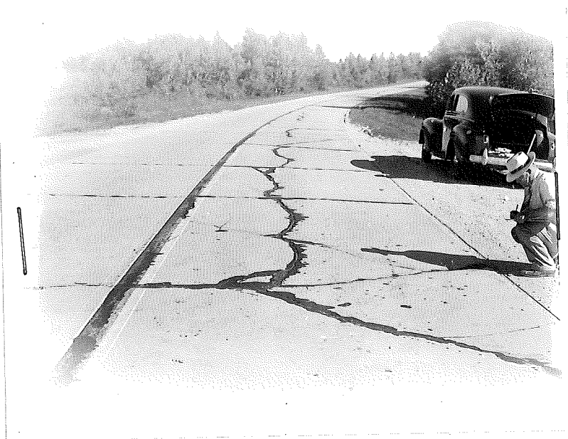
Figure 1. 49-7, C1, General view of cracking at Station 205+00. Note concrete is in excellent condition adjacent to cracks and cracks have not faulted. View looking north.
