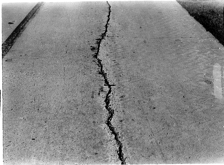
Figure 3. 49-7, C1, Close view of cracking shown in figure 2. Crack width varied from 1/2 to 3/4 inch. Note condition of concrete adjacent to crack. Looking south.
