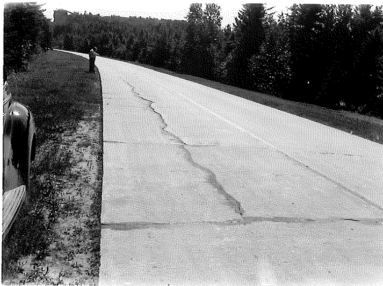
Figure 5. 49-7, C1, General view of cracking at Station 226+00 looking south. Slight faulting is noted near center of cracked area.
