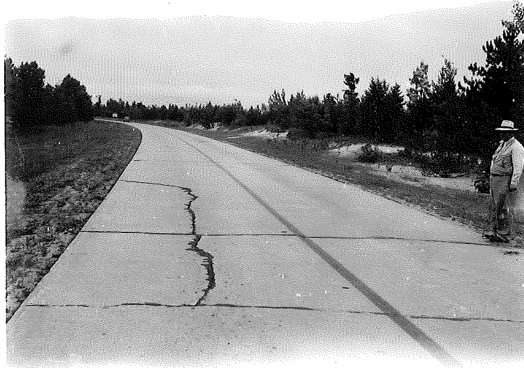
Figure 11. 49-7, C1, View at Station 384+00 looking south. Slab on side hill cut. Old road bed on left. Sand ridge on right.
