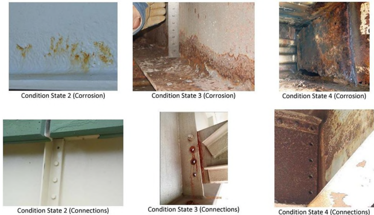
Figure 1-3. Photographs showing CS for corroded beams and connections with missing bolts (Source: MiBEIM 2017).
