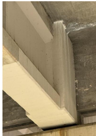
(b) Isometric view showing a leaky deck
