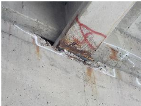
(a) Beam 3w in span 1s - undermining
