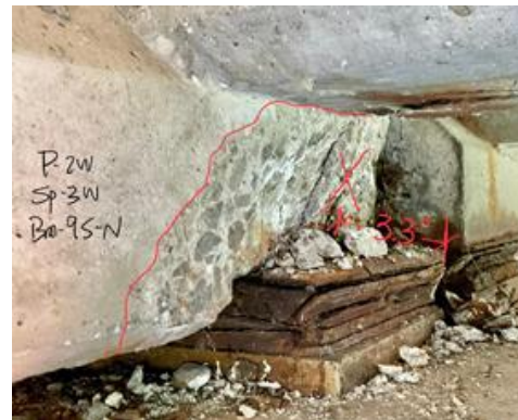
(b) Extensive spall
