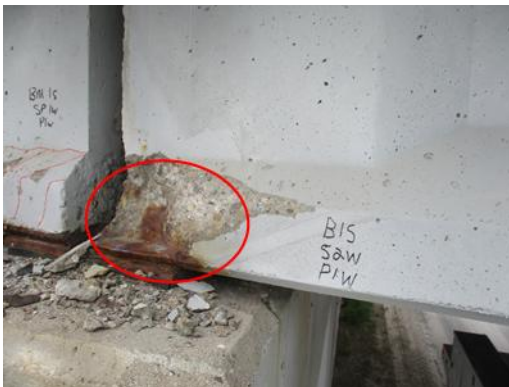
(a) Moderate spall
