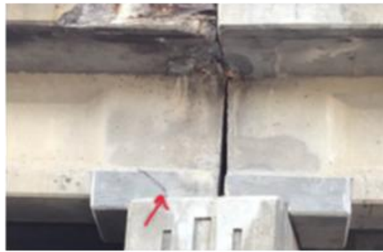
(b) Overcast at the bottom flange
