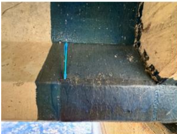
(e) Inadequate bond length leading to delamination
