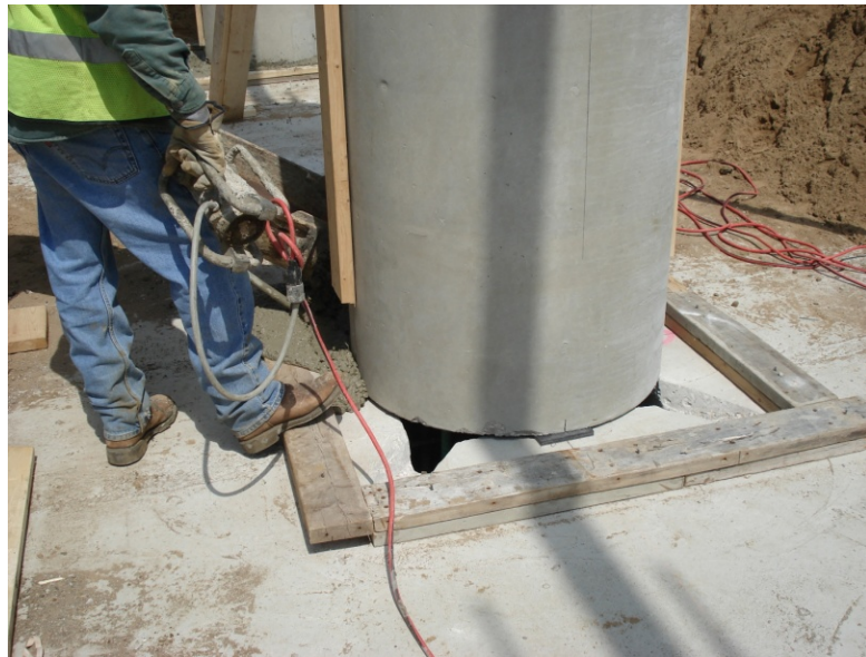
Figure 5-47. Column to footing connection with beveled void corners (Source: Photo courtesy of MDOT)
