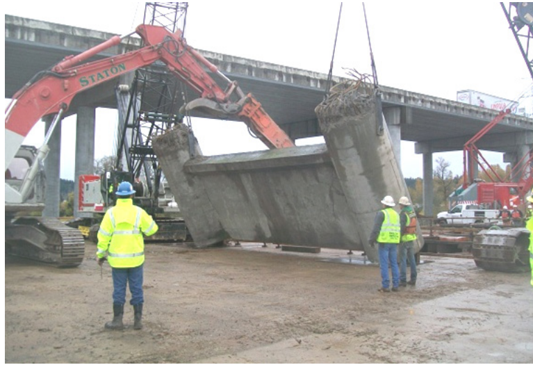
Figure 5-68. Column and pier walls are sawn off and lifted out for demolition (Source: http://www.mcgee-engineering.com )
