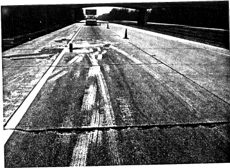
View of several spalled sympathy cracks near the beginning of section M11-1. The slope on the left shoulder is the bridge embankment. In general, the test section is on level ground.
