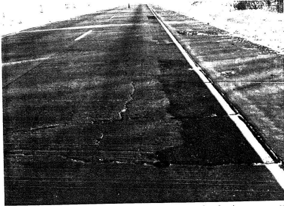
Photo #10: View of section M12-2 (East bound Galesburg) showing transverse and longitudinal cracking. Note that asphalt patching has been placed to fill in a lane shoulder dropoff of roughly one inch.
