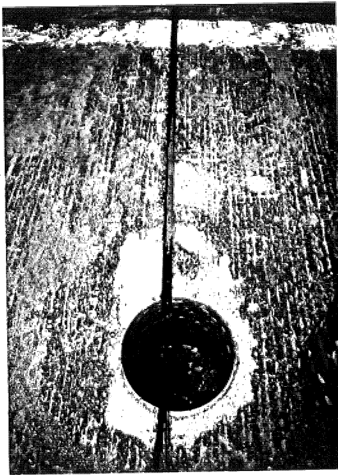
Close-up view of a core hole through a transverse joint in section MI1-2. The joint is in good condition. The OGDC is visible in the core hole. Coring water drained rapidly from the hole.
