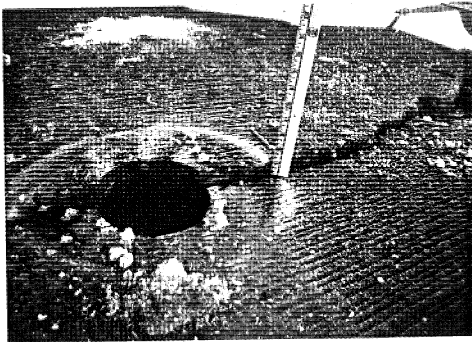
View of crack core hole in section MI2-2. Note the severe settlement of the panel with faulting of approximately one inch.
