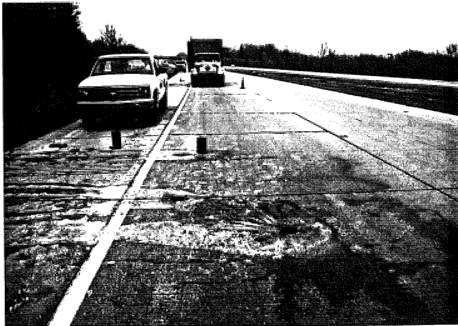
Overview of part of section MI1-2. Note the level terrain. Seen here are core holes from midpanel, crack, and joint section cores. The sympathy cracking pattern is evident.
