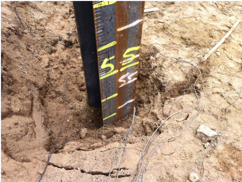
Figure 2-32 Cables of buried sensors at test pile #54 at US-131 B site
