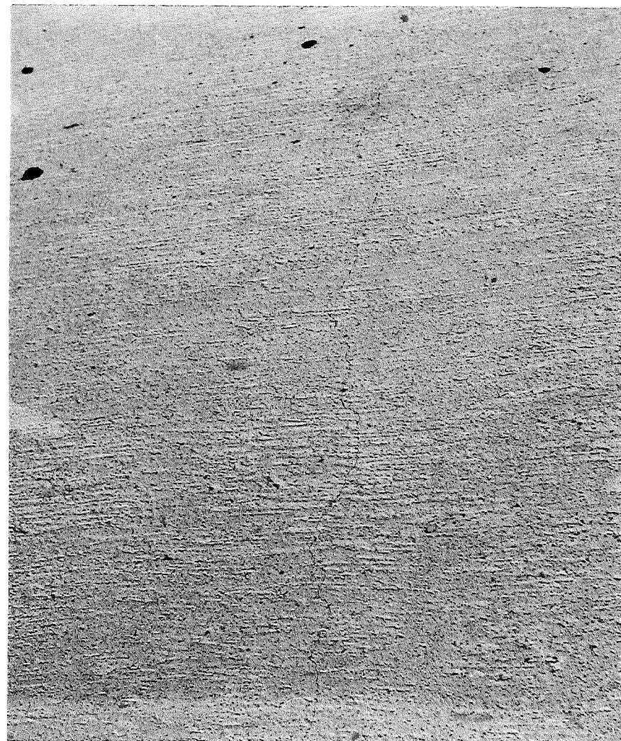
Figure 4. Second crack appeared in southbound passing lane of capped portion, F 33-54, C 4 Station 346+48, noticed in summer 1954.
