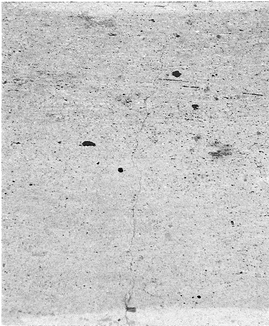
Figure 3. First crack appeared in southbound traffic lane of capped portion, F 33-54, C 4 Station 346+50 during fall 1953.
