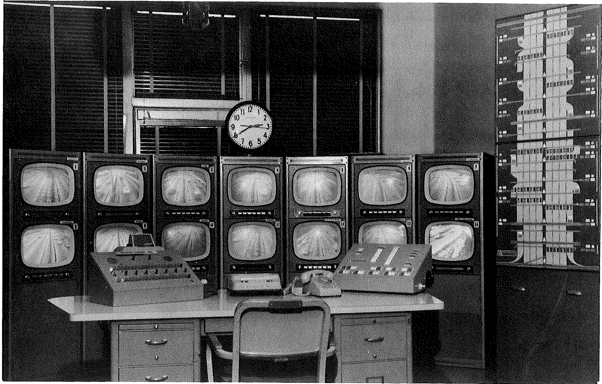
Figure 12. Television Monitoring and Confirmatory Equipment.
