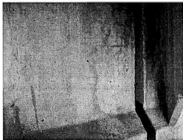
Photo 3-56. Cracks and water stain at the beam end
