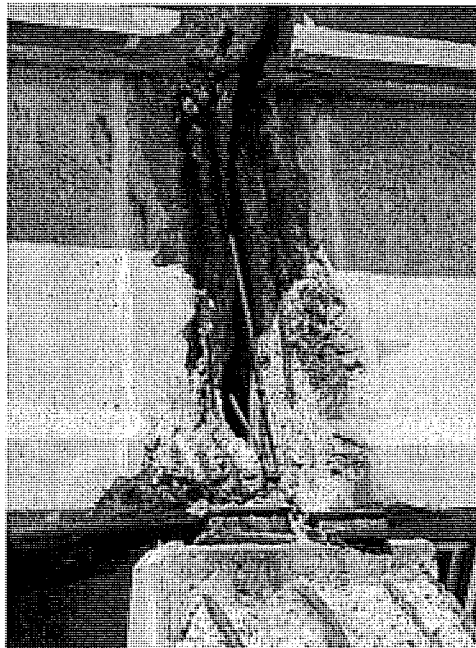
Photo 3-10. Beam-end and pier cap deterioration
