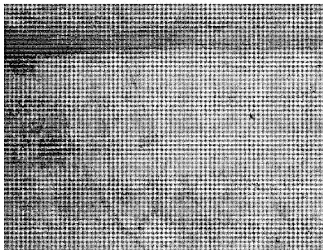
Photo 3-22. Example of hairline cracks
