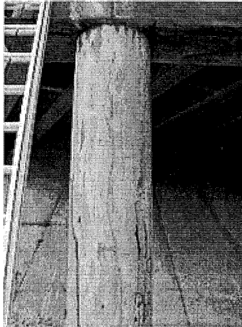
Photo 3-39. Vertical cracks at column S4 of the pier W1
