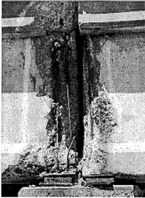
Photo 3-6. Severe deterioration of beam-end
