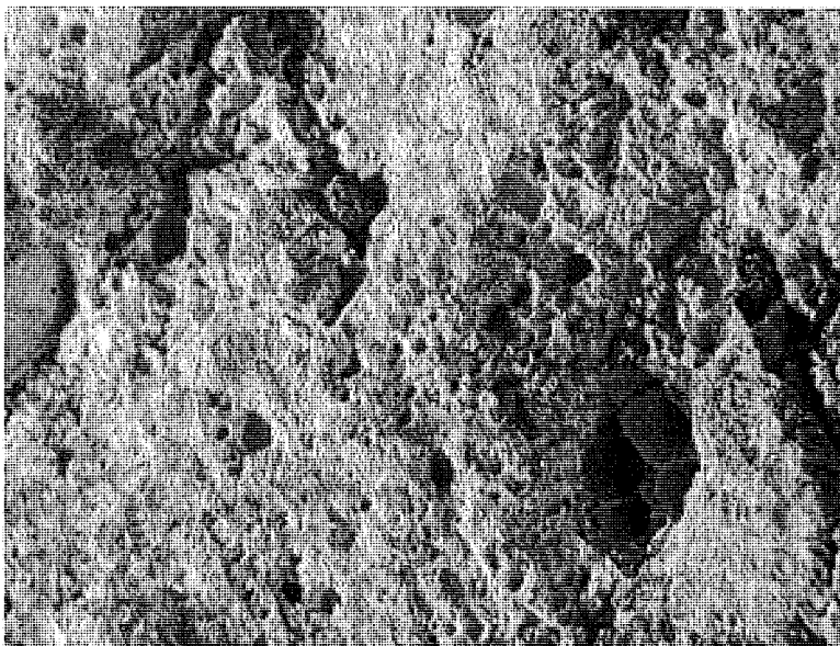
Photo 11-11. Wire brushed surface profile at 20x magnification, non-depressed region
