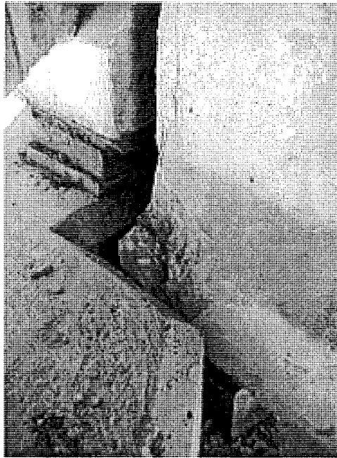
Photo 3-57. Cracks, spalls and exposed reinforcement at some of the beam-ends
