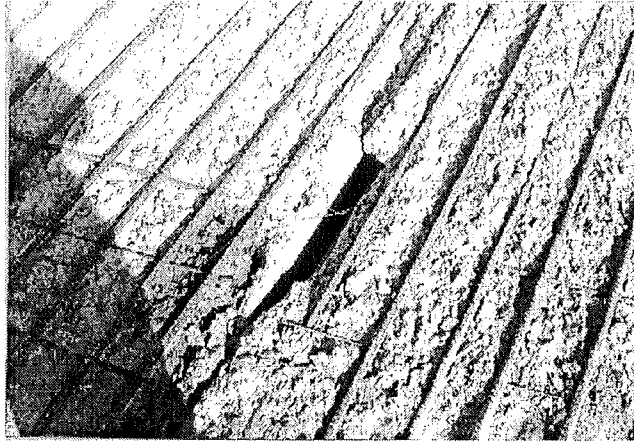
Photo 3-44. Hole at the deck West approach
