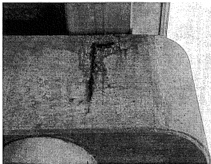
Photo 3-51. Spall with exposed reinforcement at pier S1 under beam W1
