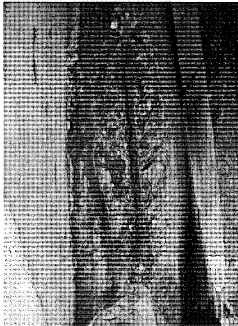
Photo 3-37. Beam-end exhibiting significant deterioration
