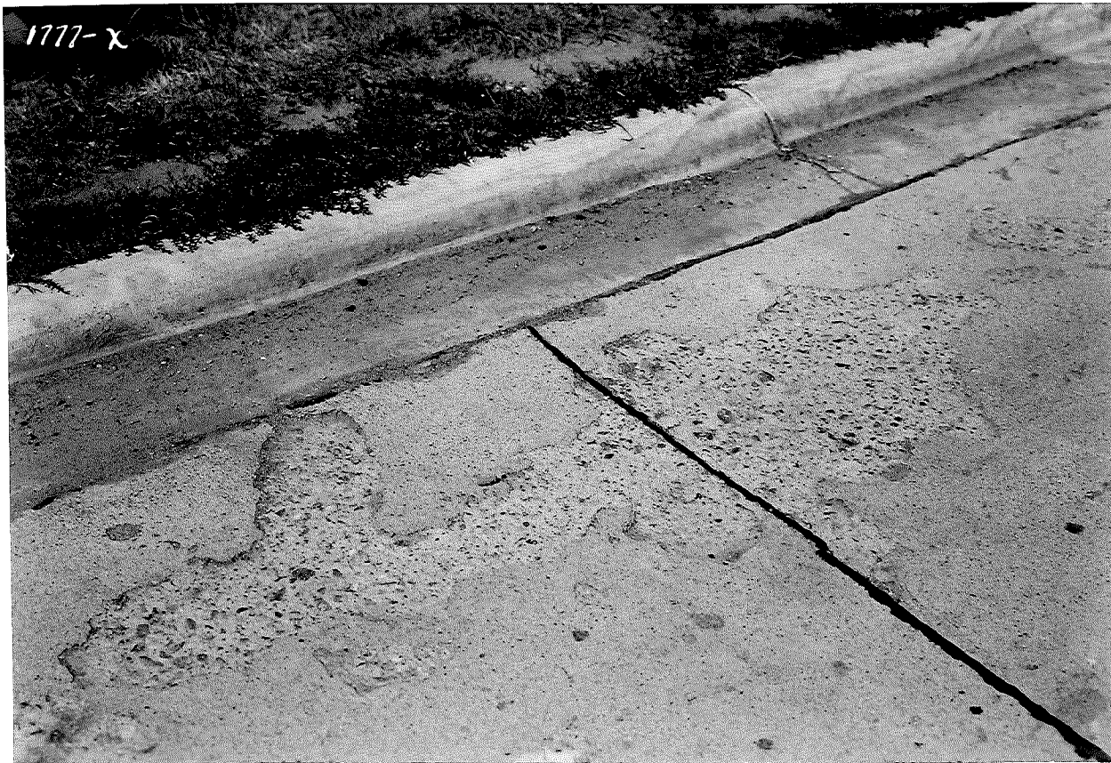
Figure 1 - Typical Scaling of Concrete Pavement
