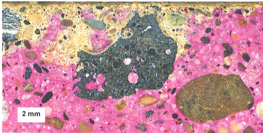
Figure 21. Part of phenolphthalein stained polished slab from F1, showing variation of carbonation along the surface.
