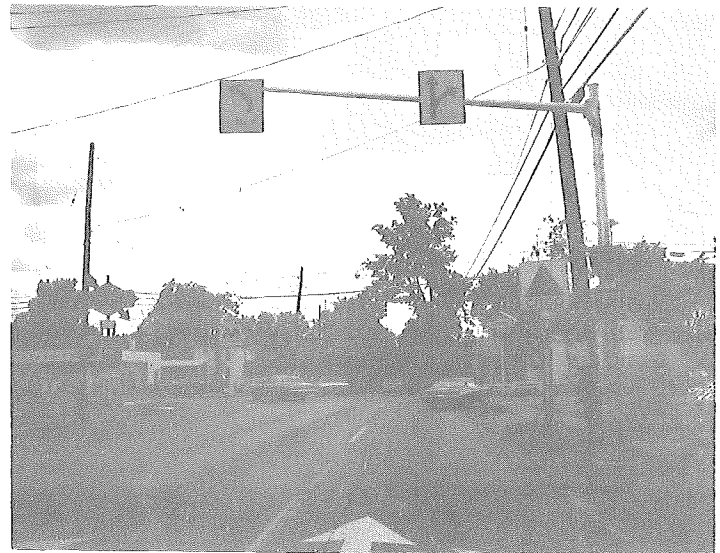
SECTIONAL POLE CANTILEVER ON BL-94 (EATON ST.) @ AUSTIN ST., CITY OF ALBION. DATE OF ERECTION: 9-9-69.
