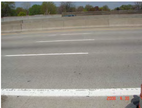
Figure 6. Stainless steel reinforced bridge deck surface, S03 of 63103, I-696 over Lenox Road, Ferndale, Michigan, in April 2008.
