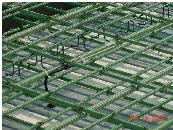
Figure 7. Rohrback Cosasco Corrosometer Model 650-T-50 corrosion probe tied to top mat reinforcement of R12-3 of 33045.
