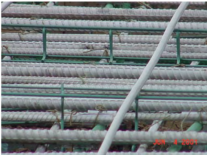
Figure 10. The solid stainless steel reinforcement installed on westbound I-496, R12-4 of 33045, has a dull grey color.
