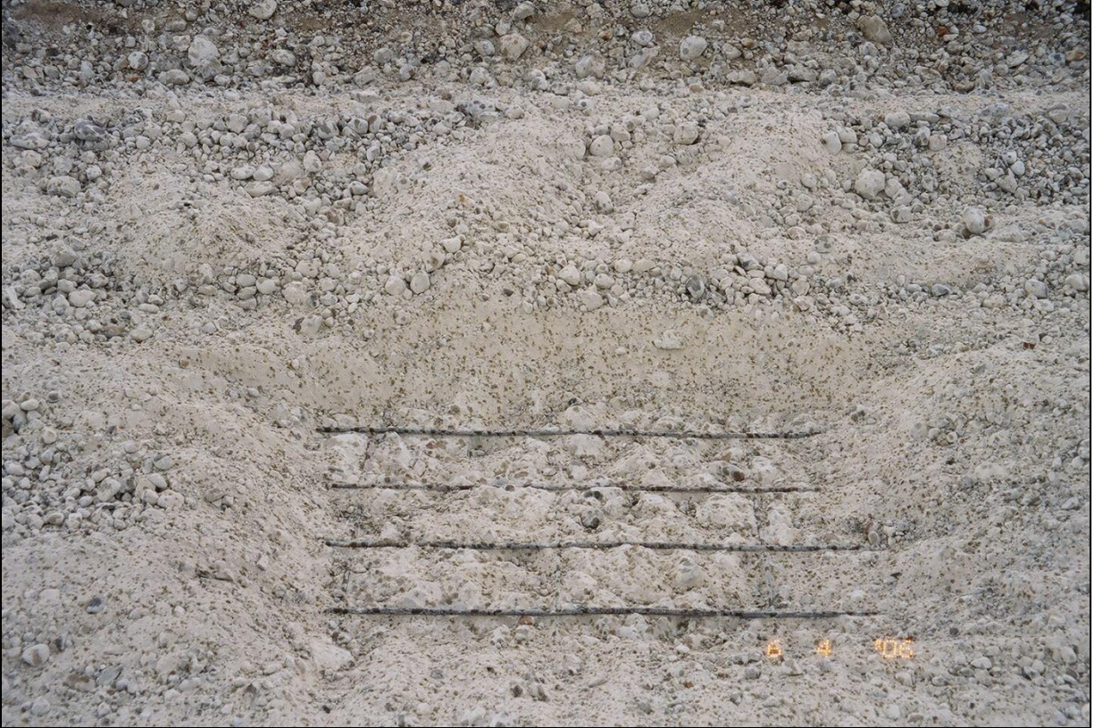
Figure 33. Photo of rubblized PCC for which the elastic modulus back-calculated from deflection basins is low, ranging from 25,000 to 50,000 psi
