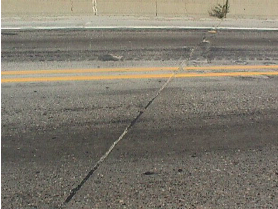
Figure 3-25. Destruction of joint
