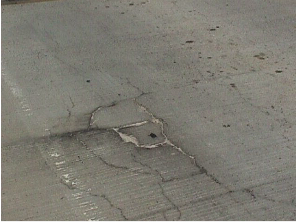
Figure 3-4. Pattern cracking (large)
