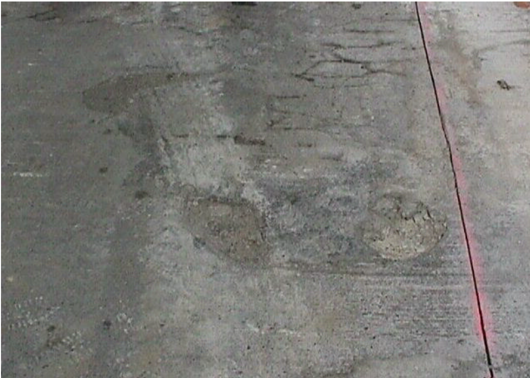
Figure 3-3. Pattern cracks (large)
