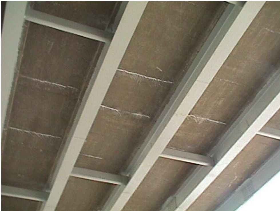
Figure 3-11. Transverse cracks (bottom of the deck), caused by restraint shrinkage
