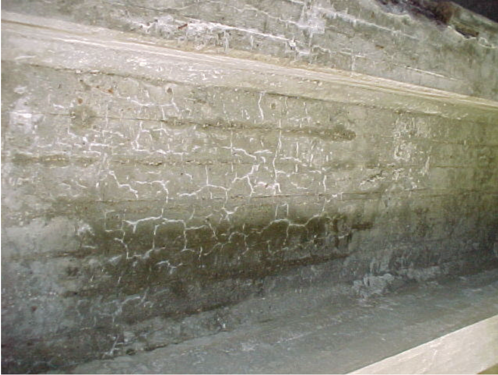
Figure 3-2. Pattern cracks (bottom of the deck)
