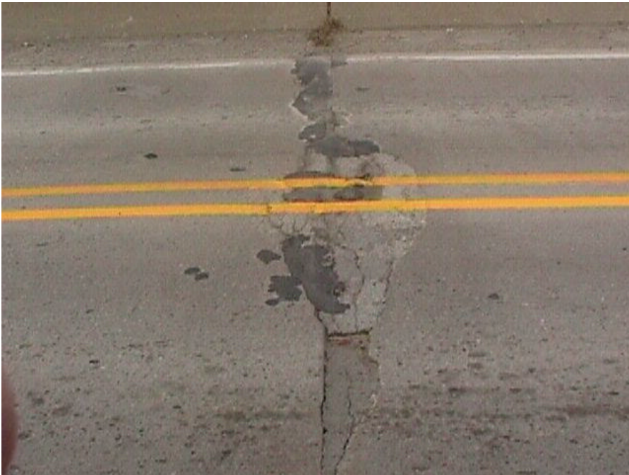
Figure 3-26. Destruction close to joint
