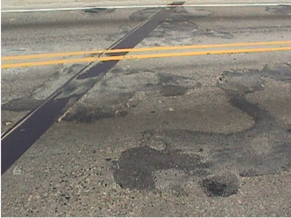
Figure 3-27. Destruction close to joint
