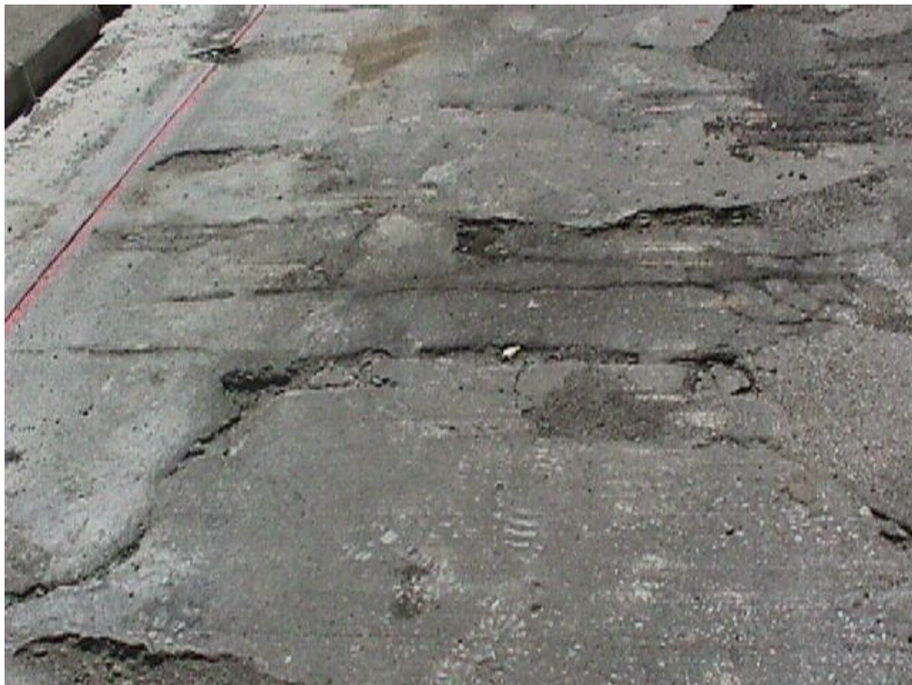
Figure 3-21. Potholes with local erosion of material, located on the line of bigger crack
