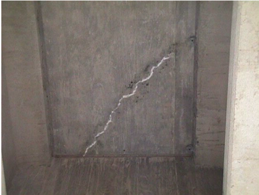
Figure 3-13. Diagonal crack close to support (bottom of the deck)
