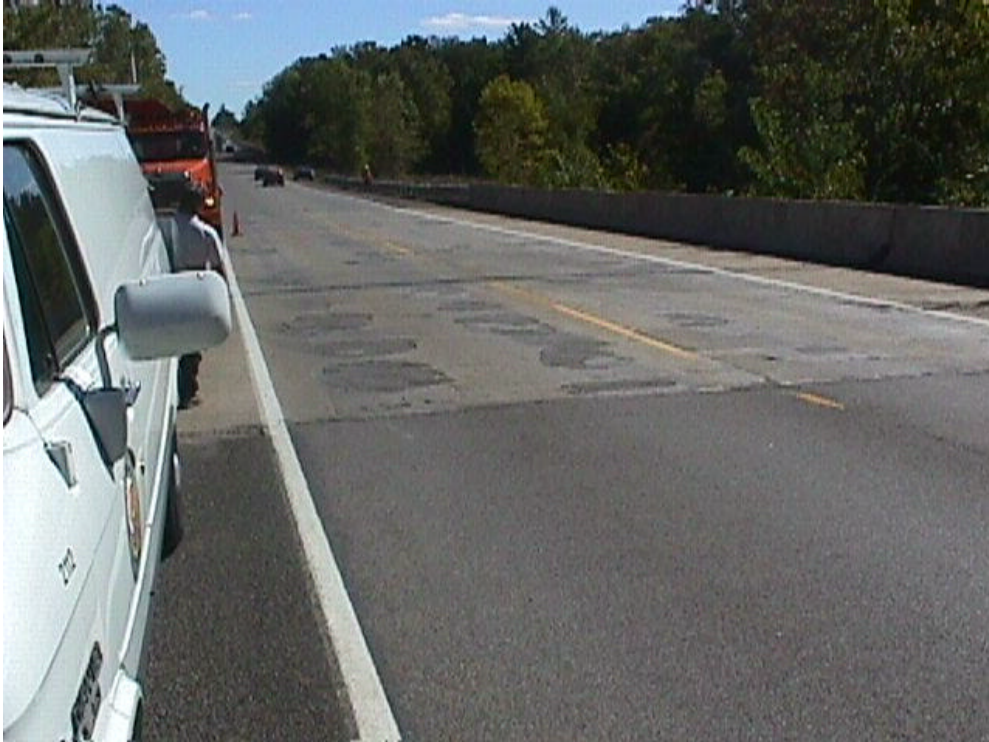
Figure 3-22. Potholes following pattern of wheels
