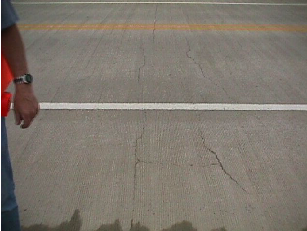
Figure 3-10. Transverse cracks, caused by restraint shrinkage
