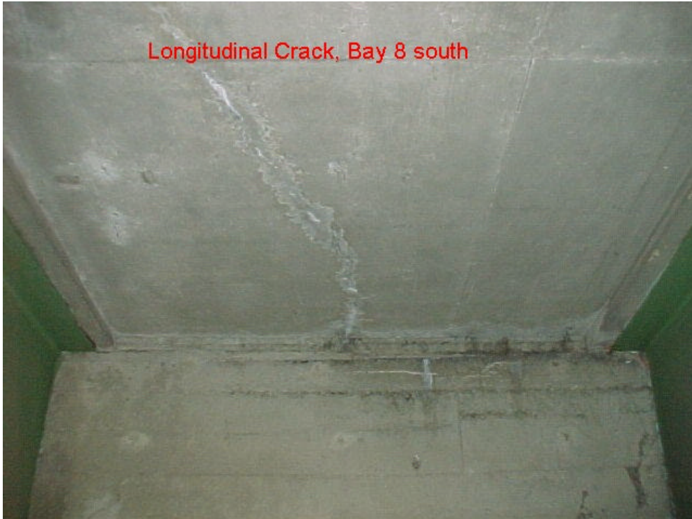
Figure 3-8. Longitudinal crack (bottom of the deck)
