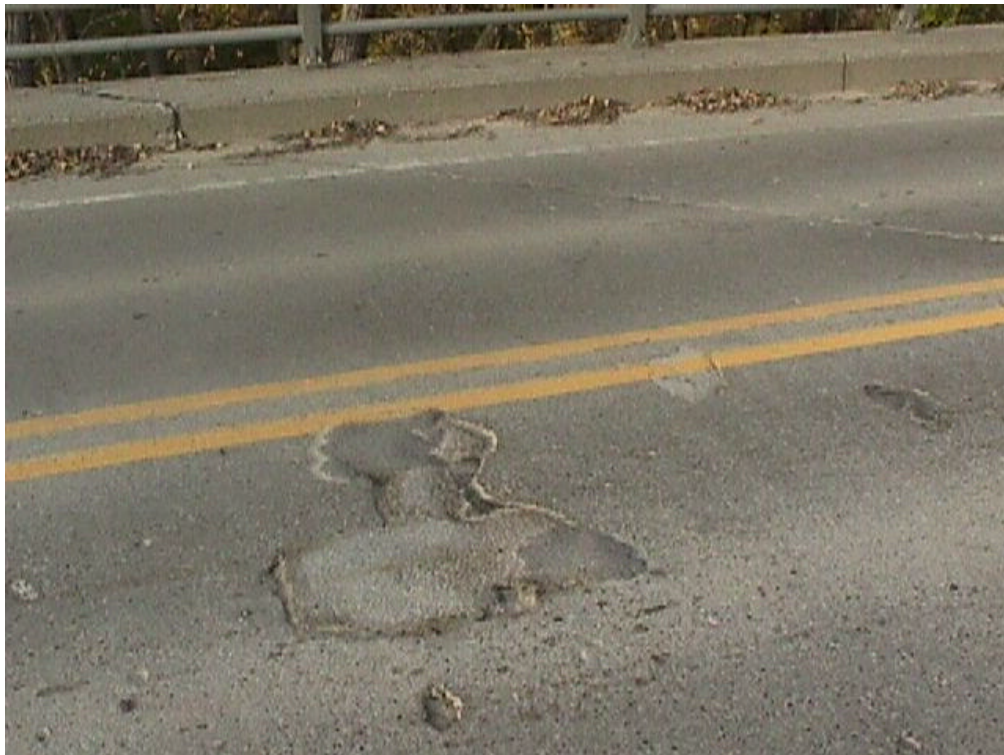
Figure 3-23. Potholes in latex overlay
