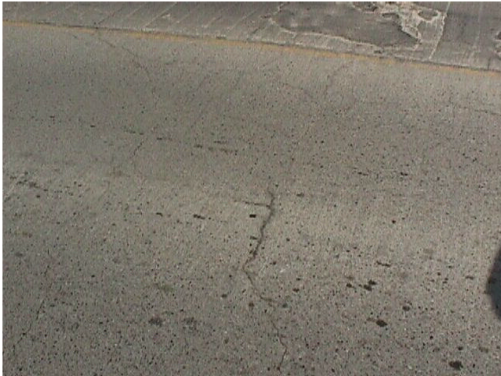
Figure 3-1. Craze cracks (top of the deck)
