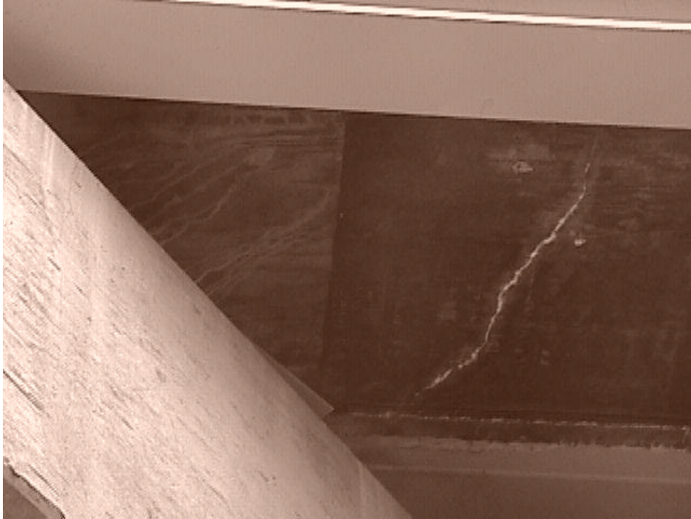
Figure 3-14. Diagonal crack close to joint (bottom of the deck)
