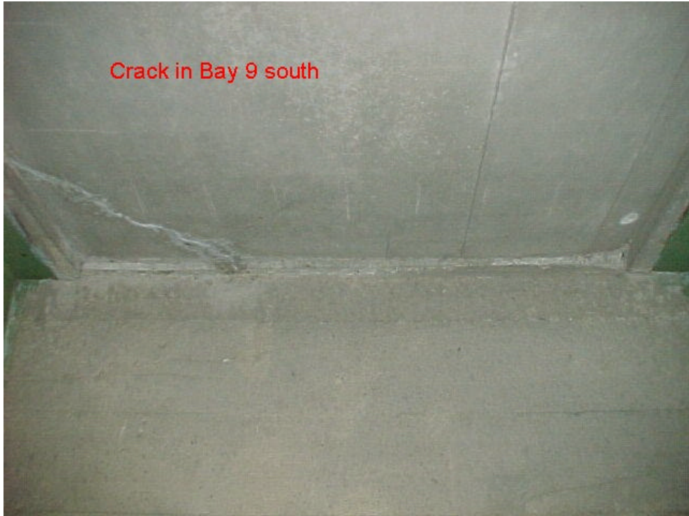
Figure 3-12. Diagonal crack close to support (bottom of the deck)
