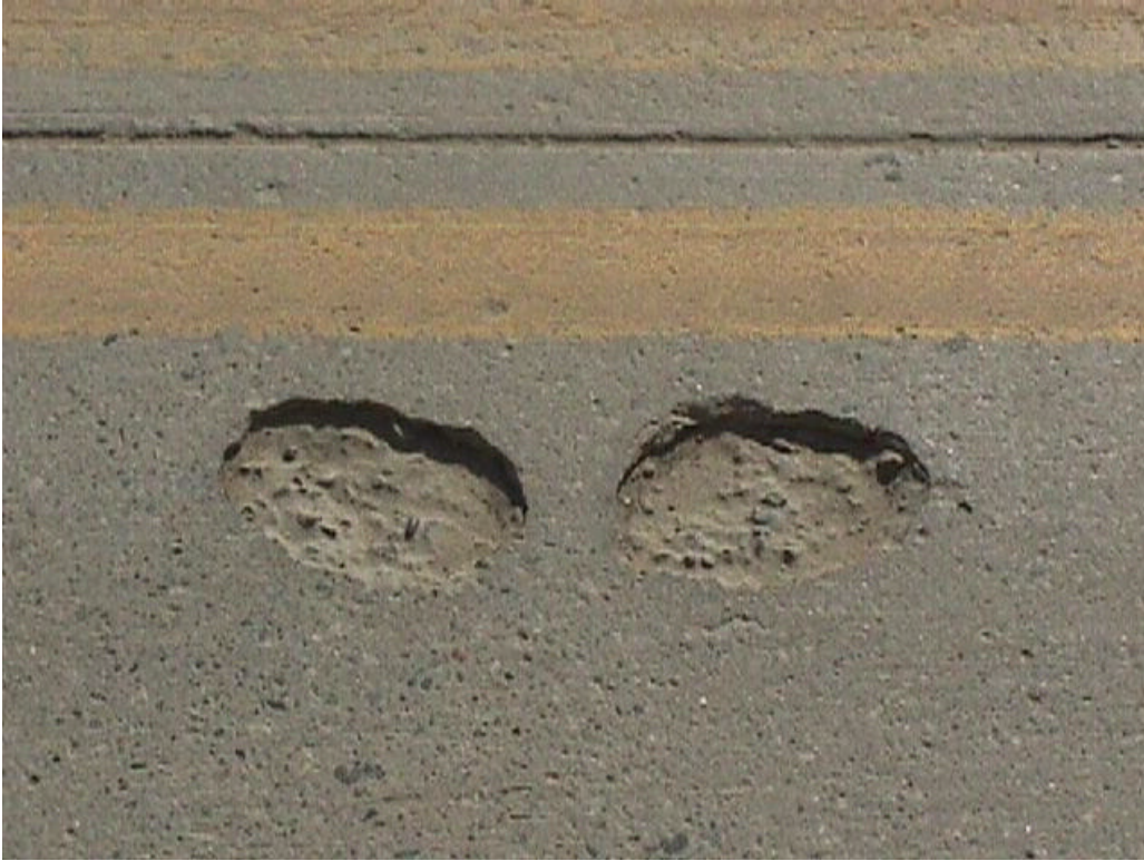
Figure 3-24. Potholes in latex overlay
