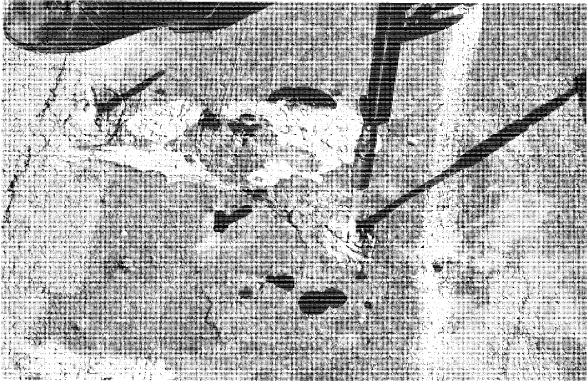
Figure 7. Close-up before and after views of epoxy injection of a delaminated area. Note stoppered vent port and fissures where epoxy escaped.
